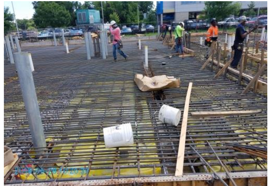
Figure 13. Construction crews completing the framing of the new fire station on Read Boulevard, June 28, 2018.
