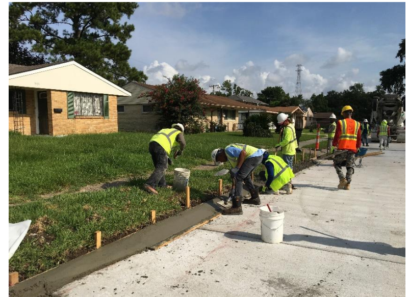
Figures 5 & 6. Crews repairing damaged concrete panels on Lacour Monique Street in Algiers (above). Installation of new curbs on Pittari Street in Algiers (below).
