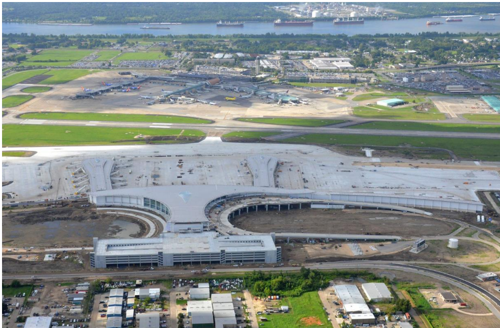
Figure 19. Most recent aerial image of construction site of the new airport terminal.
