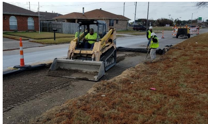
Figure 3 & 4. Crews working on Michoud Boulevard Reconstruction Project (above), and crews replacing damaged concrete panels on Bullard Avenue between Hayne Boulevard and Chef Menteur Highway (below).
