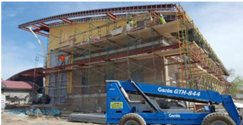
Figures 14 & 15. Rendering of proposed police station (above) and recent construction progress photo (below).
