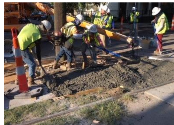
Figure 9. Crews beginning forming and placing Americans with Disabilities Act-compliant ramps on the
