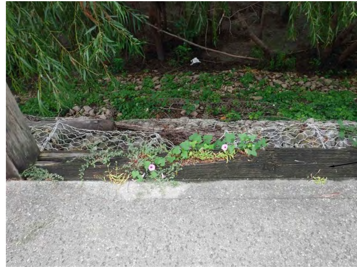
ROTTEN TIMBERS. THIS EXAMPLE HAS VEGETATION
