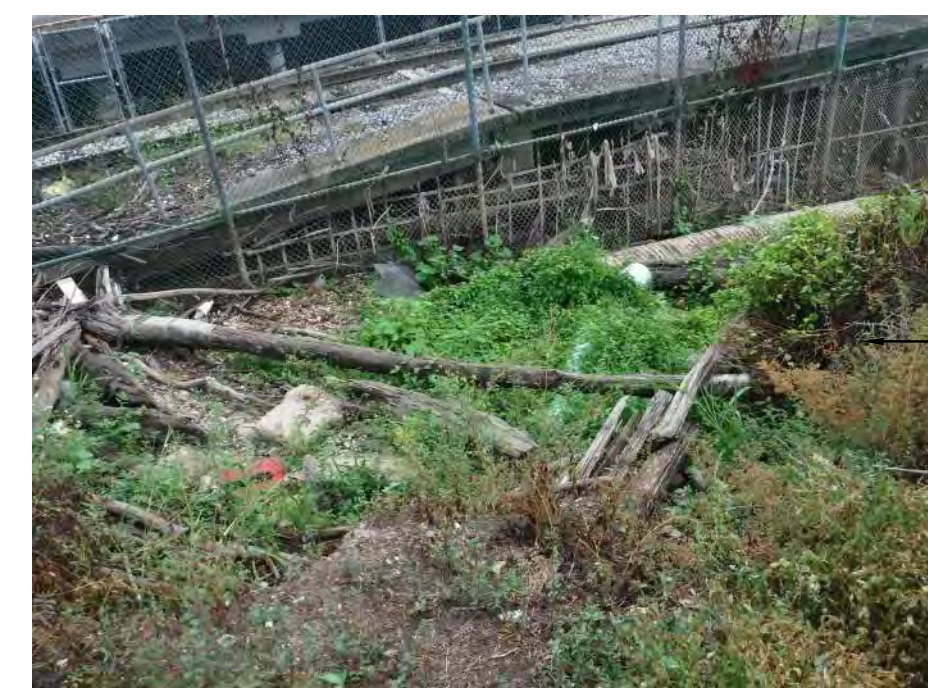
AREA OF SEVERE EROSION
