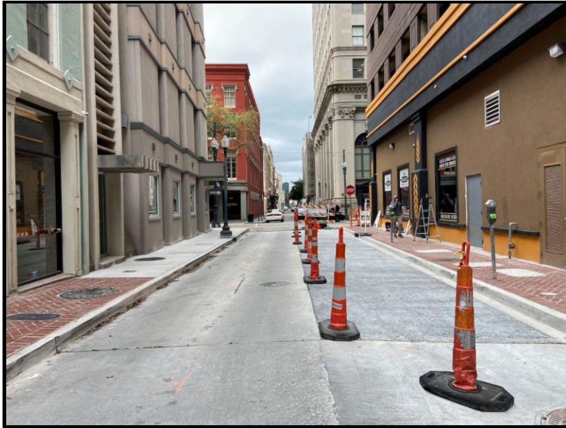
Figure 8: Pervious Street Paving in the CBD
