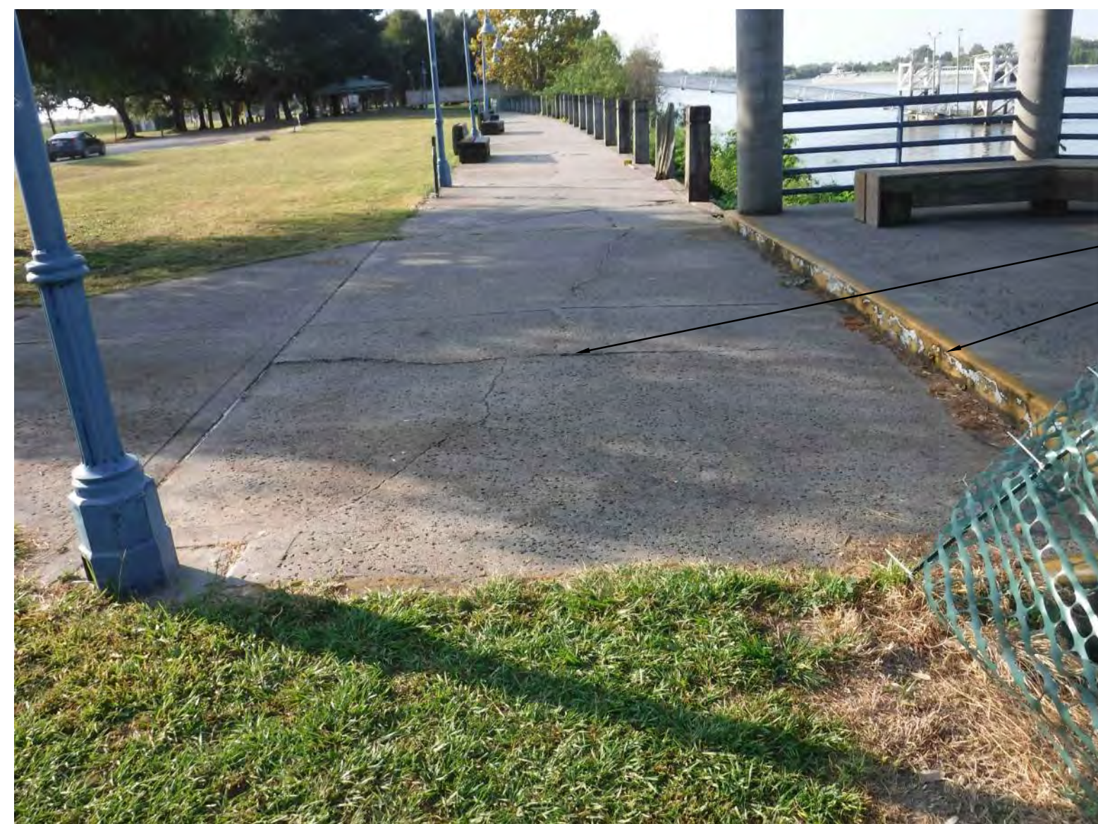
MINOR CRACKS IN SIDEWALK STEP UP TO PAVILION EXCEEDS ALLOWABLE 7" MAXIMUM
