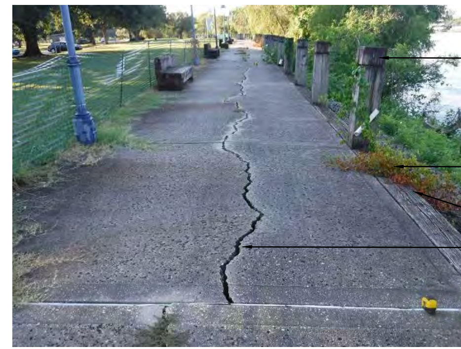
TOPS OF TIMBER BOLLARDS ARE ROTTEN, TYP. SOME ARE LOOSE TIMBER BULKHEAD SUBSIDING DOWN BANK SLOPE, TYPICAL CONDITION TIMBERS ROTTEN WHERE INDICATED CRACK ALONG SIDEWALK
