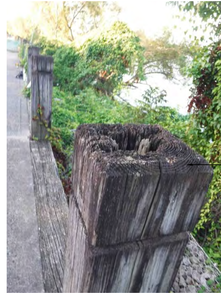
EXAMPLE OF ROTTEN TIMBER BOLLARD AT TOP
