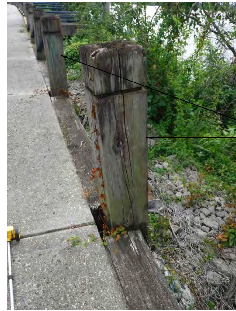
TIMBER BOLLARDS ROTTEN AT TOP, AND LOOSE
