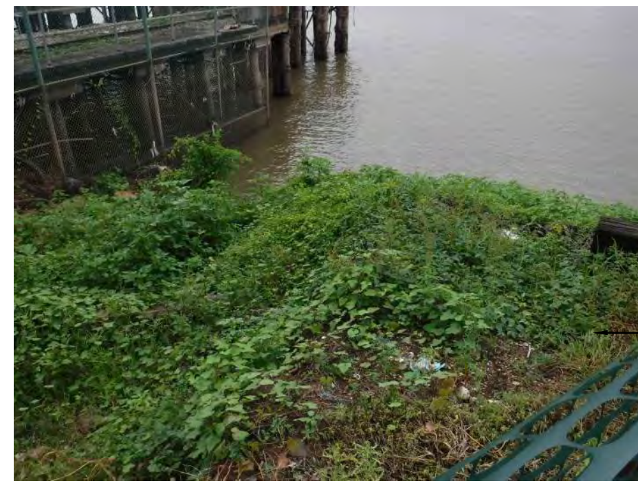
AREA OF SEVERE EROSION
