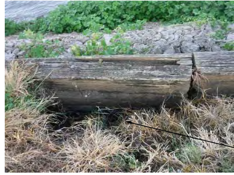
PORTION OF WASHOUT BEHIND TIMBERS
