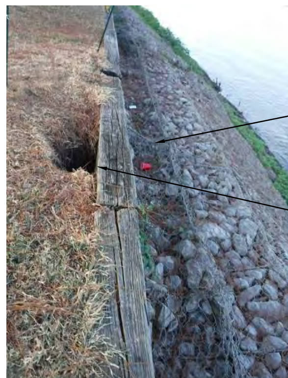
ENTIRE ROW OF TOP GABIONS MISSING/DAMAGED
