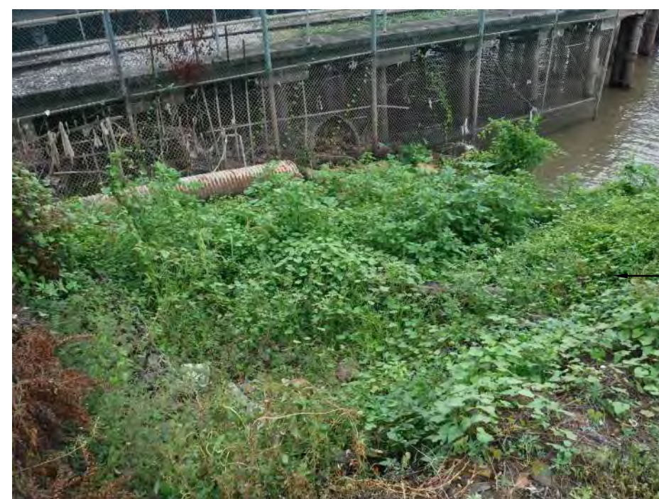
AREA OF SEVERE EROSION
