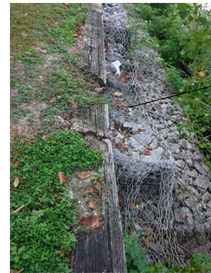
DAMAGED GABION BASKETS
