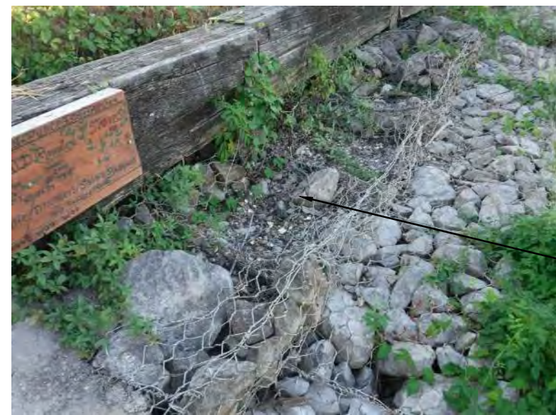
MISSING/DAMAGED TOP ROW OF GABIONS
