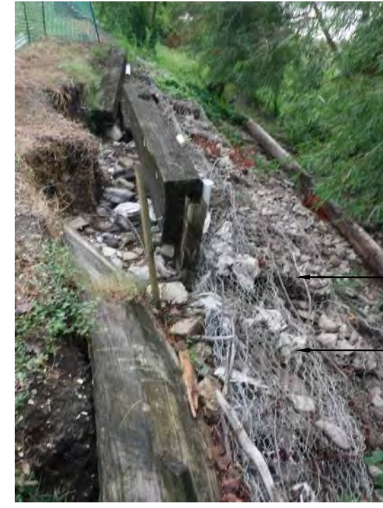
BULKHEAD FAILURE AT ZONE 5 EMPTIED/DAMAGED GABIONS
