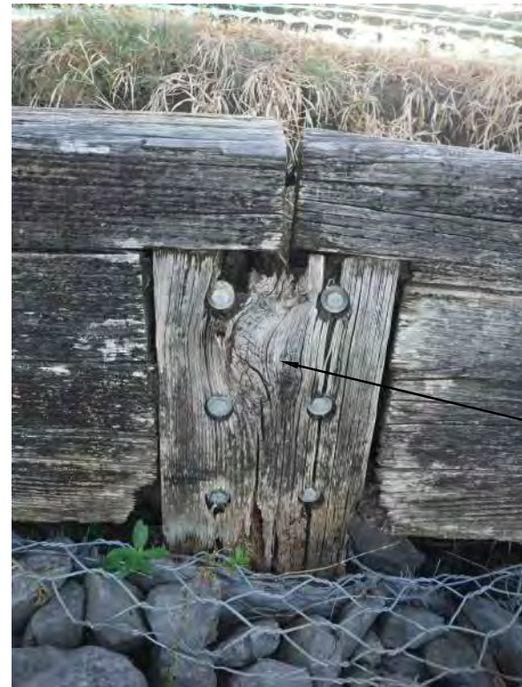
ROTTEN VERTICAL SUPPORT BETWEEN HORIZONTAL TIMBERS
