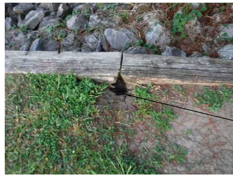
HOLE BEHIND ROTTEN VERTICAL SUPPORT
