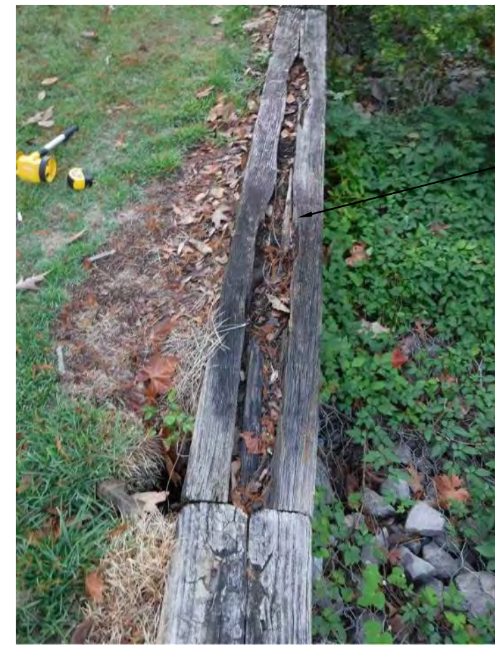
EXAMPLE OF ROTTEN TIMBER
