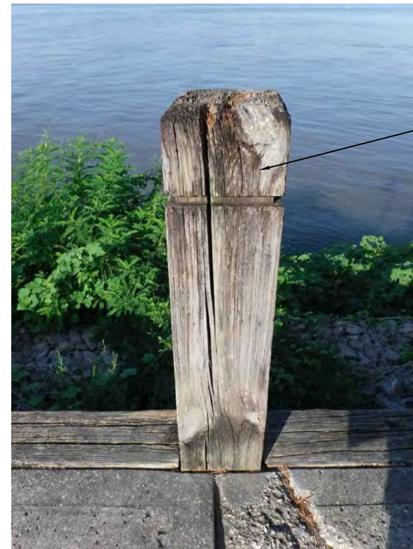
EXAMPLE OF ROTTEN AND/OR LOOSE TIMBER BOLLARD
