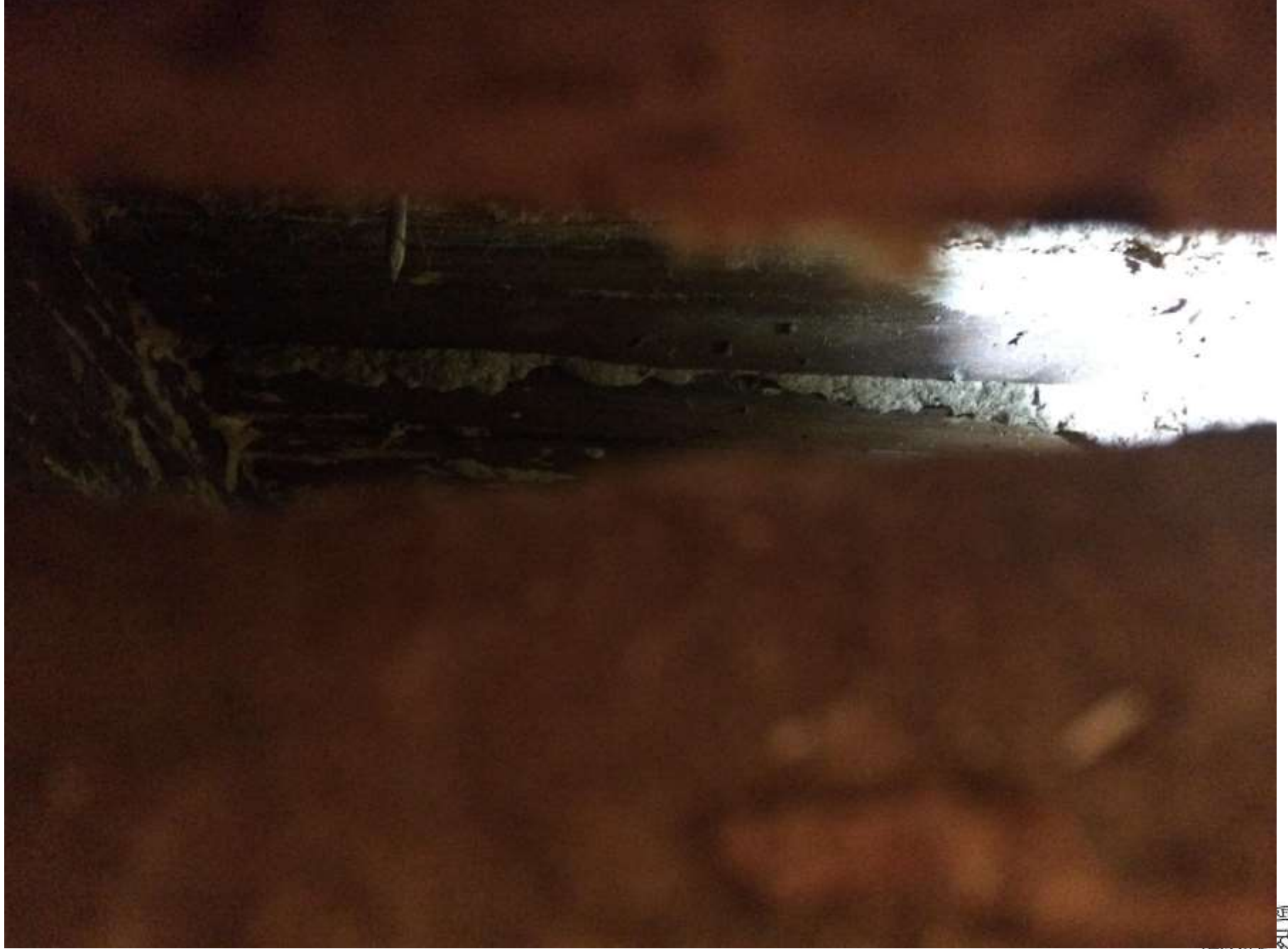
1030 Orleans – Cavity below existing window sill
