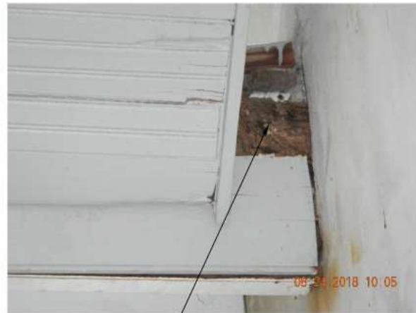
FLOOR JOIST DAMAGE
