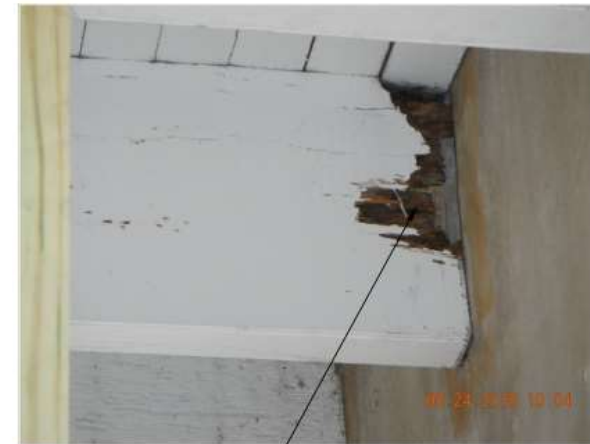
FLOOR JOIST DAMAGE
