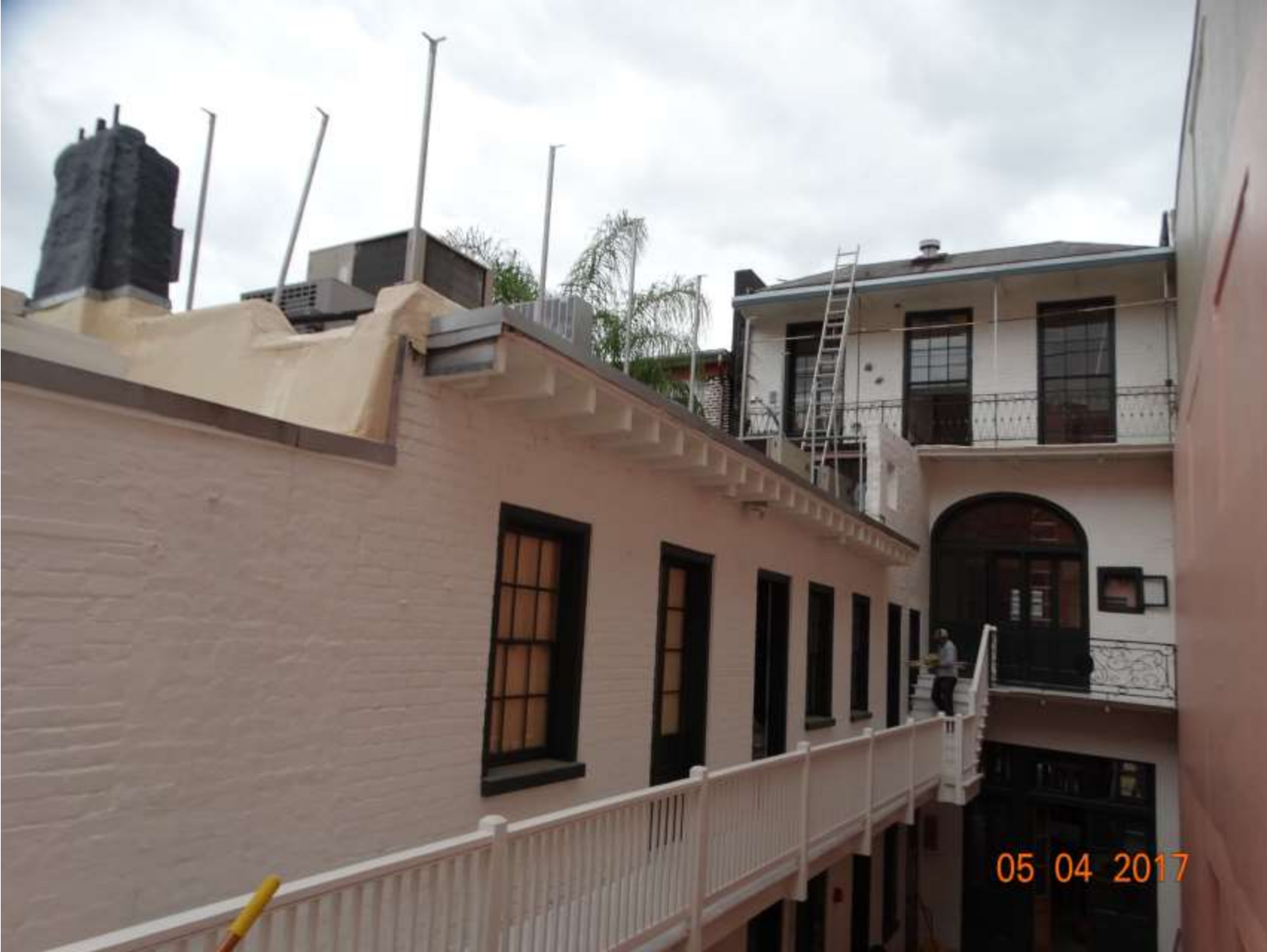
217 Bourbon – Millwork Discrepancies – Second Floor Doors Joined
