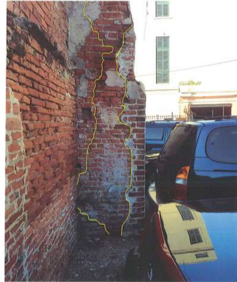
Photo #6-View of cracked section of southwest wall
