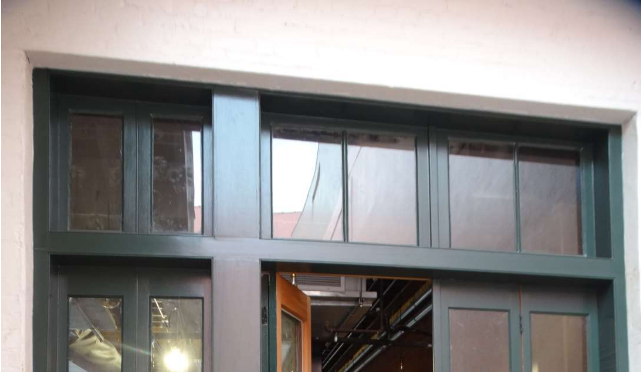
217 Bourbon – Millwork Discrepancies – First Floor Doors Under Fanlight – As Built Condition
