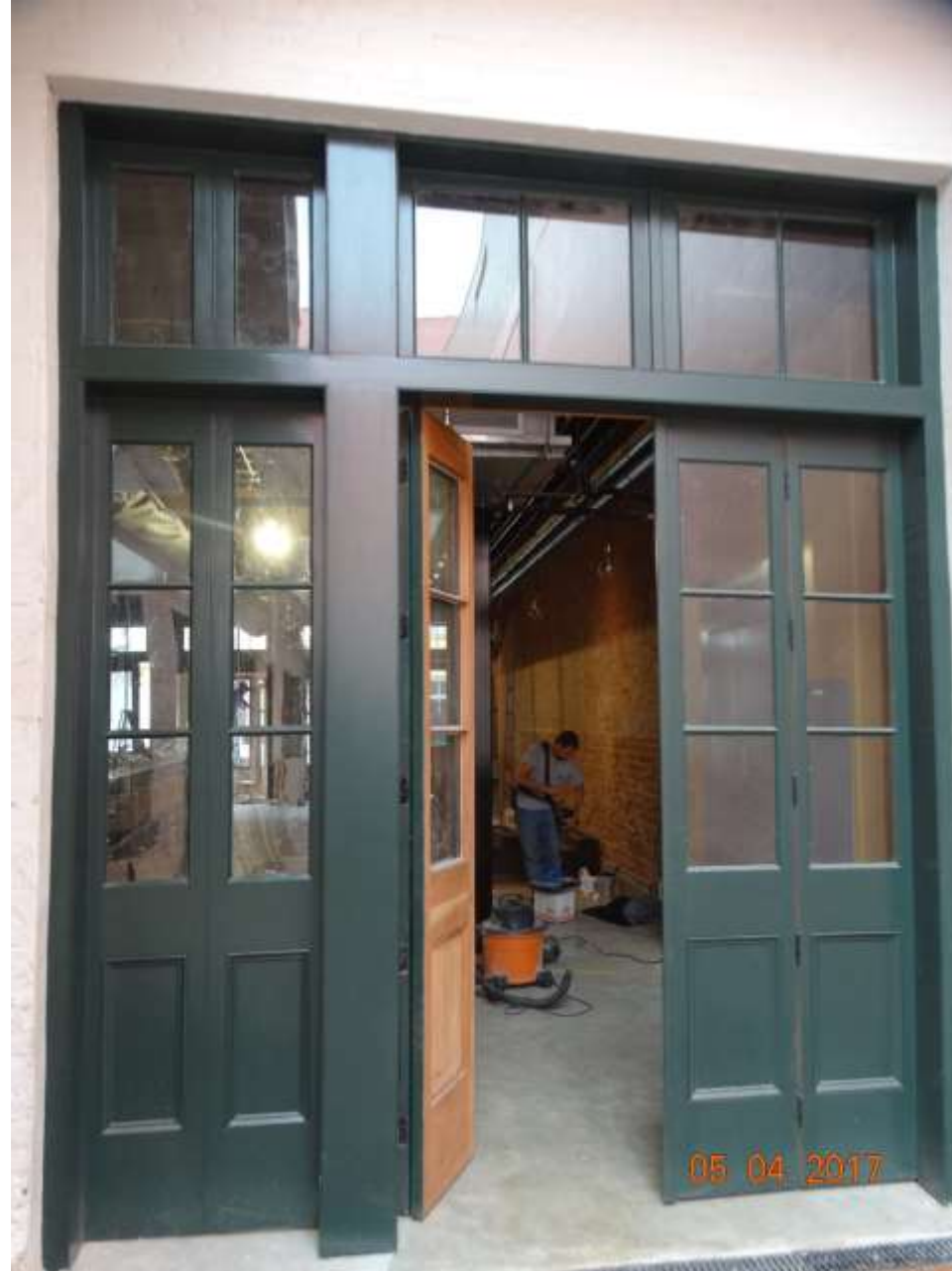
217 Bourbon – Millwork Discrepancies – First Floor Doors Under Fanlight – As Built Condition
