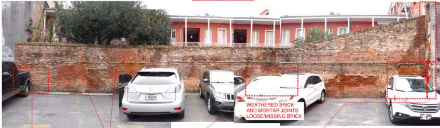
WEATHERED BRICK AND MORTAR JOINTS
