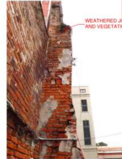
WEATHERED JOINTS & BRICK, SOME MISSING/LOOSE
