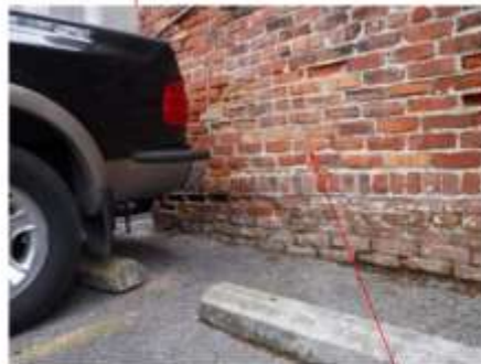
WEATHERED BRICK AND MORTAR JOINTS
