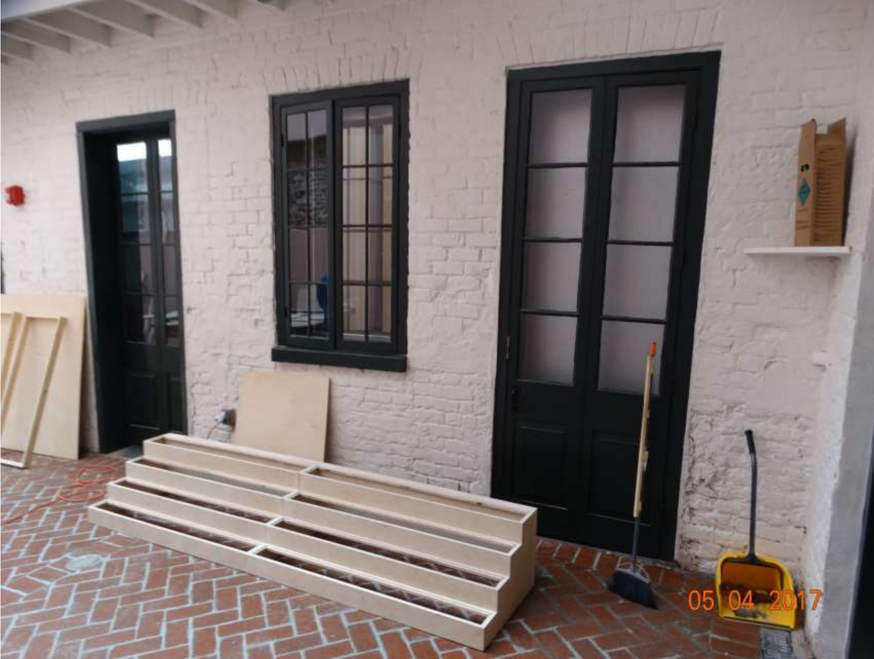
217 Bourbon – Millwork Discrepancies – Doors Joined and Out swinging
