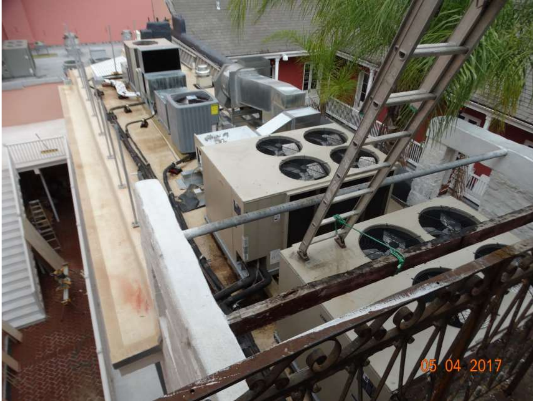
217 Bourbon – As-built Mechanical Equipment
