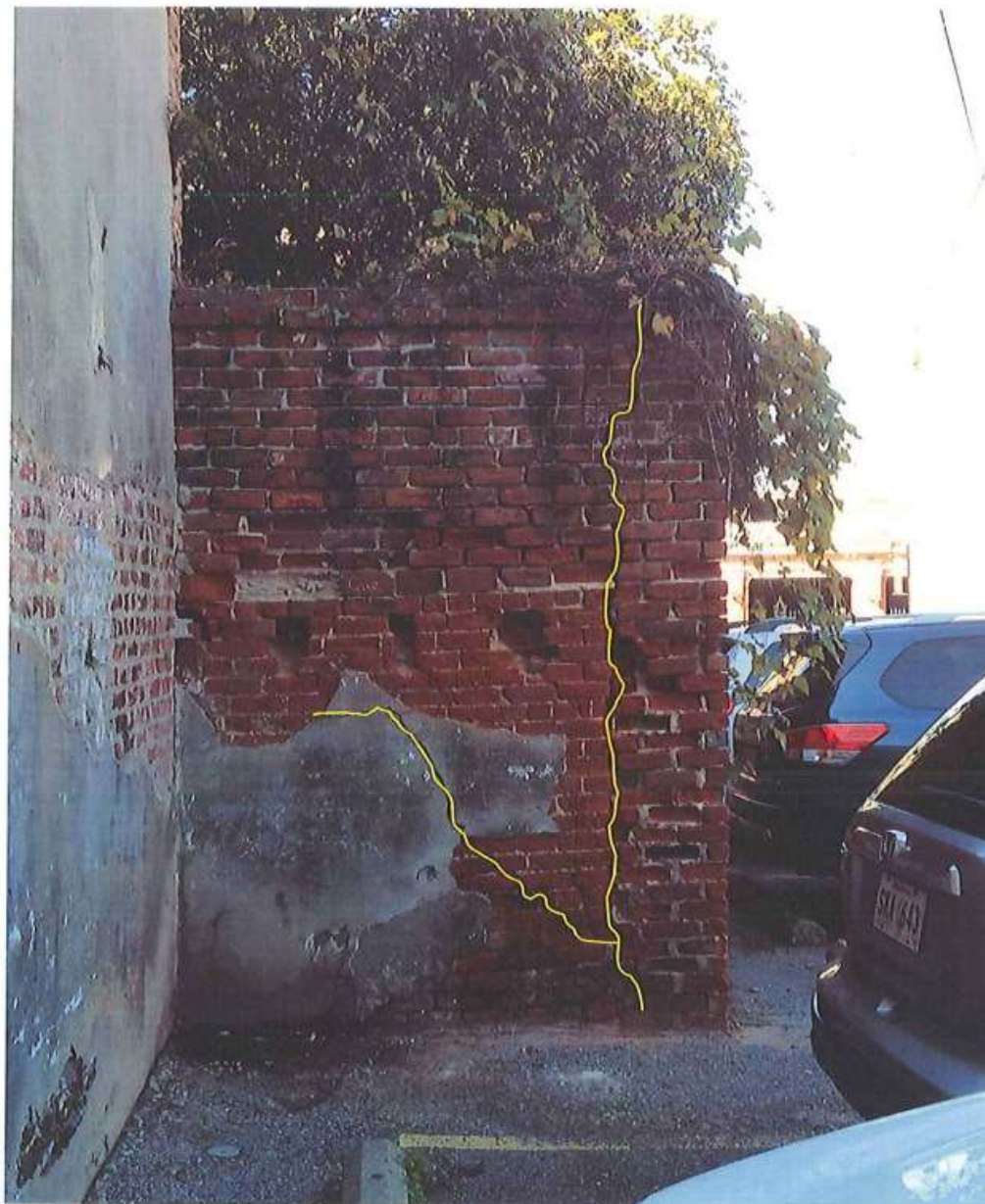
Photo #5-View of cracked section of southwest wall
