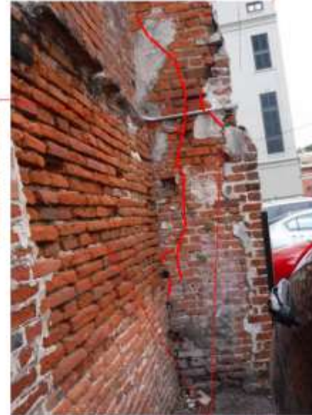
WEATHERED JOINTS & BRICK, SOME MISSING/LOOSE, VEGETATION
