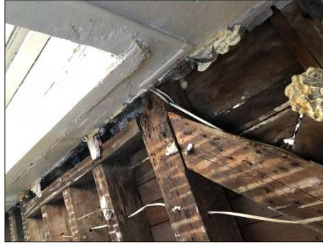
Third floor framing condition at north wall above window 203
