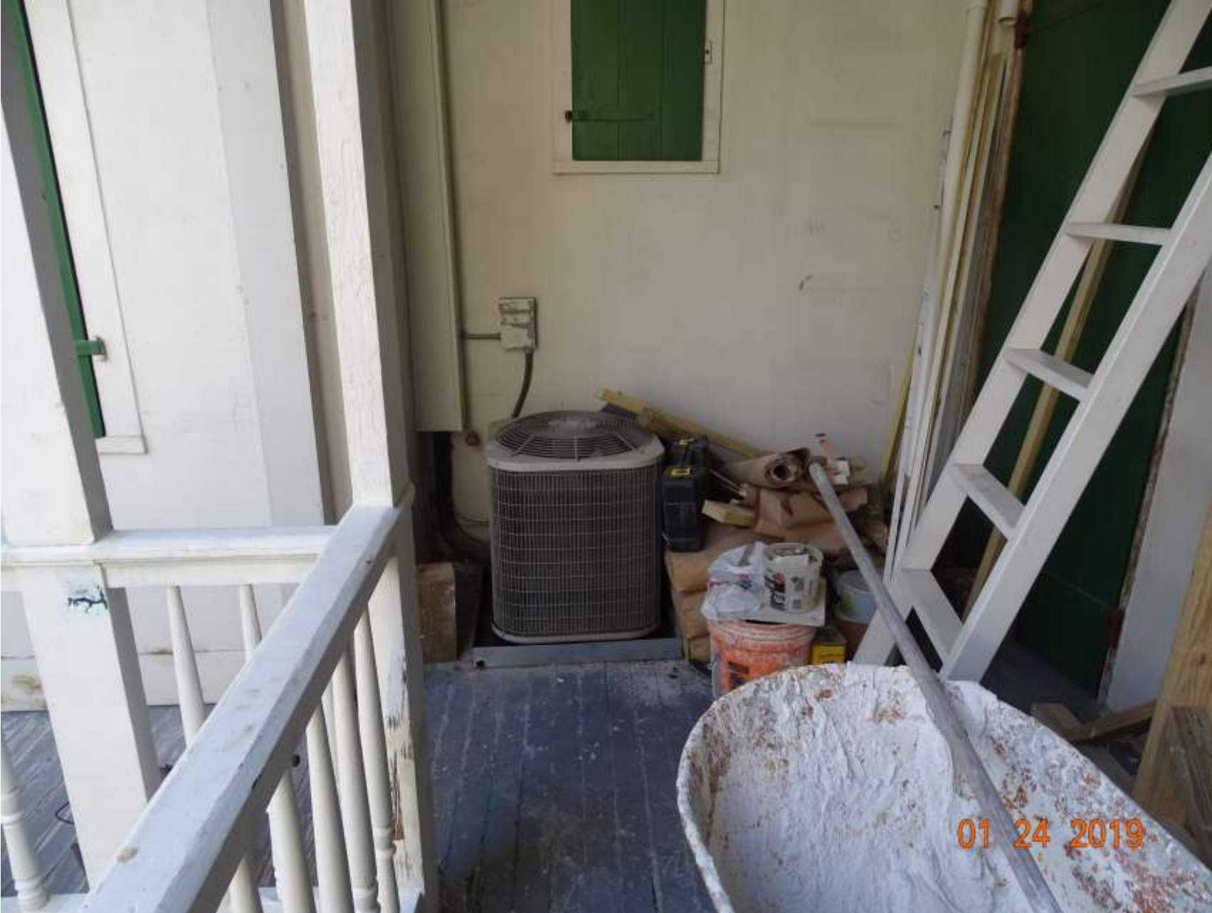
836 St. Peter – Existing Balcony HVAC Unit
