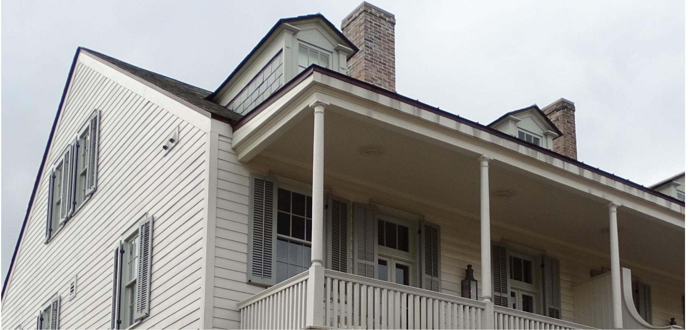
822 Barracks – No Gutters or Downspouts installed
