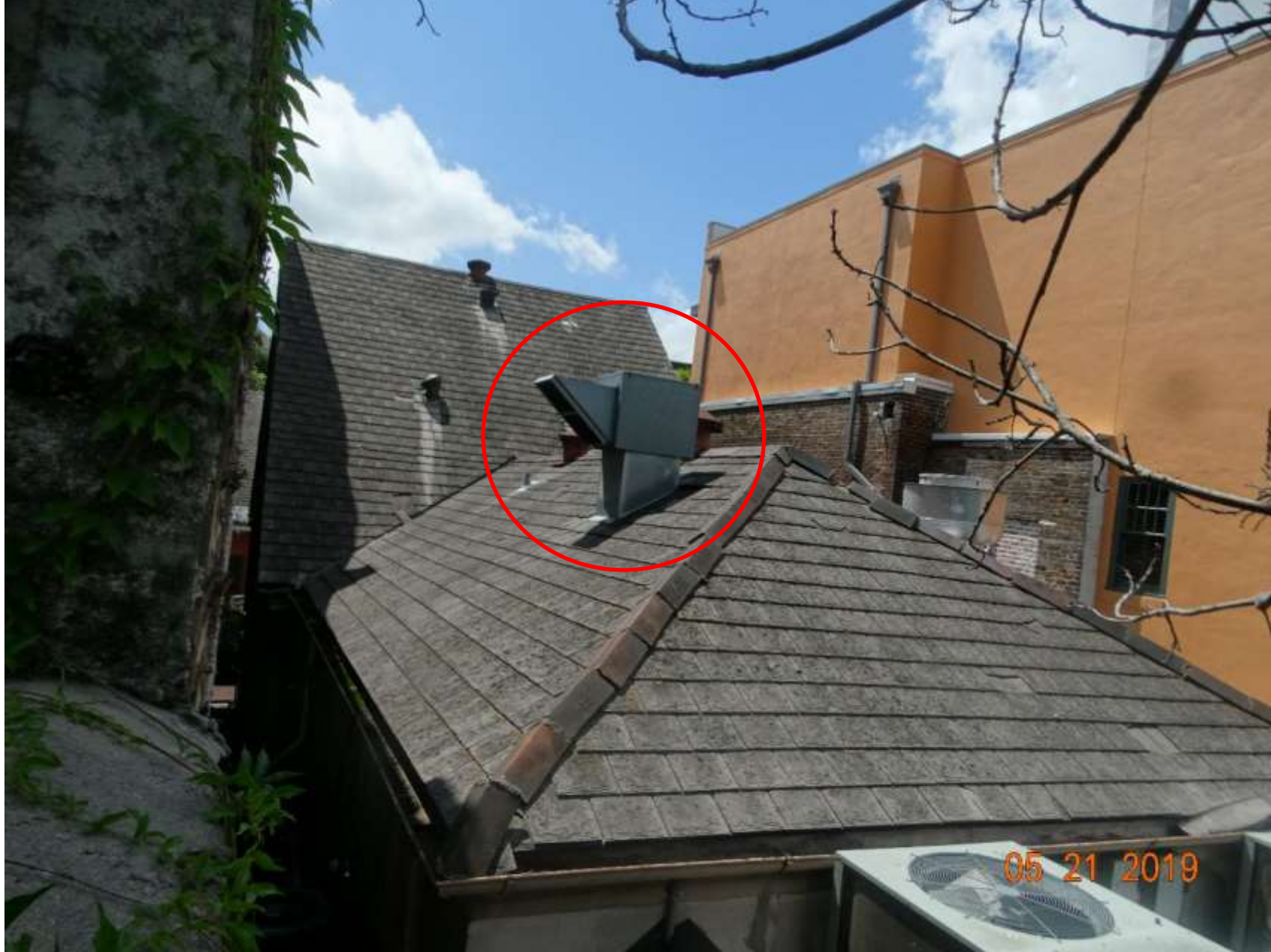
417-19 Bourbon – Previously Existing Air Intake
