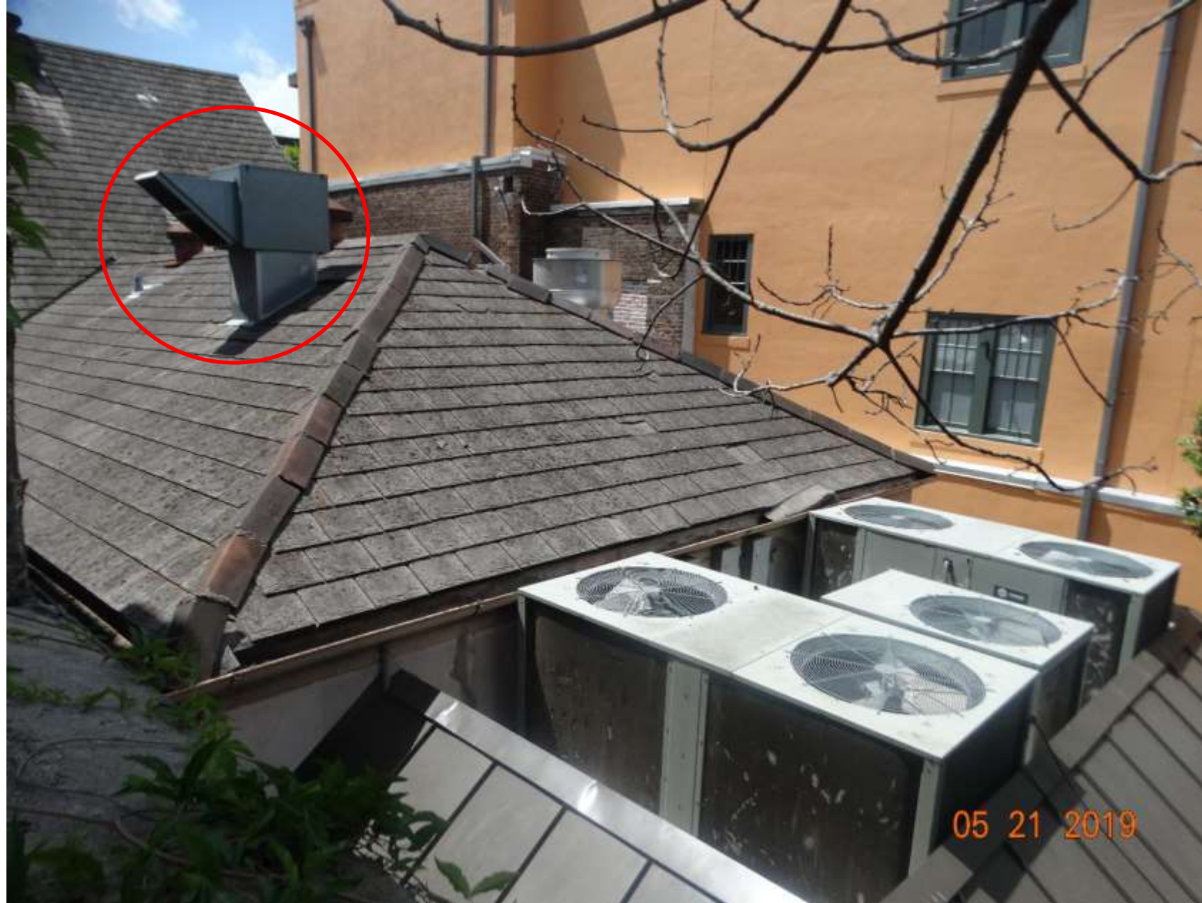
417-19 Bourbon – Previously Existing Air Intake
