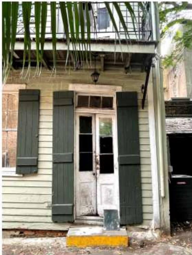
Photo 1: View of Settled Corner
