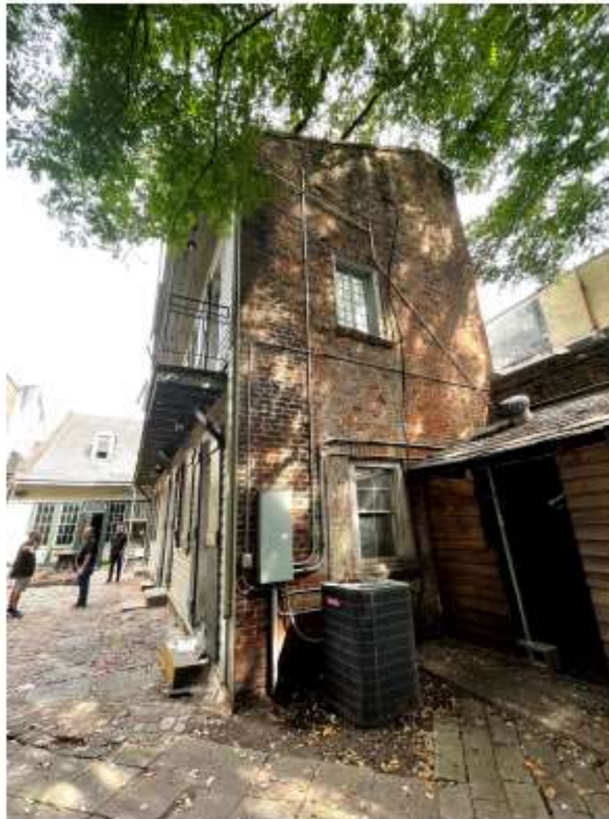
Photo 3: View of Settled Corner
