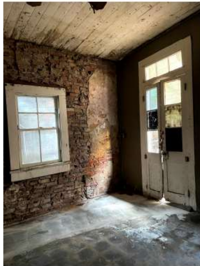
Photo 2: Interior View of Settled Corner
