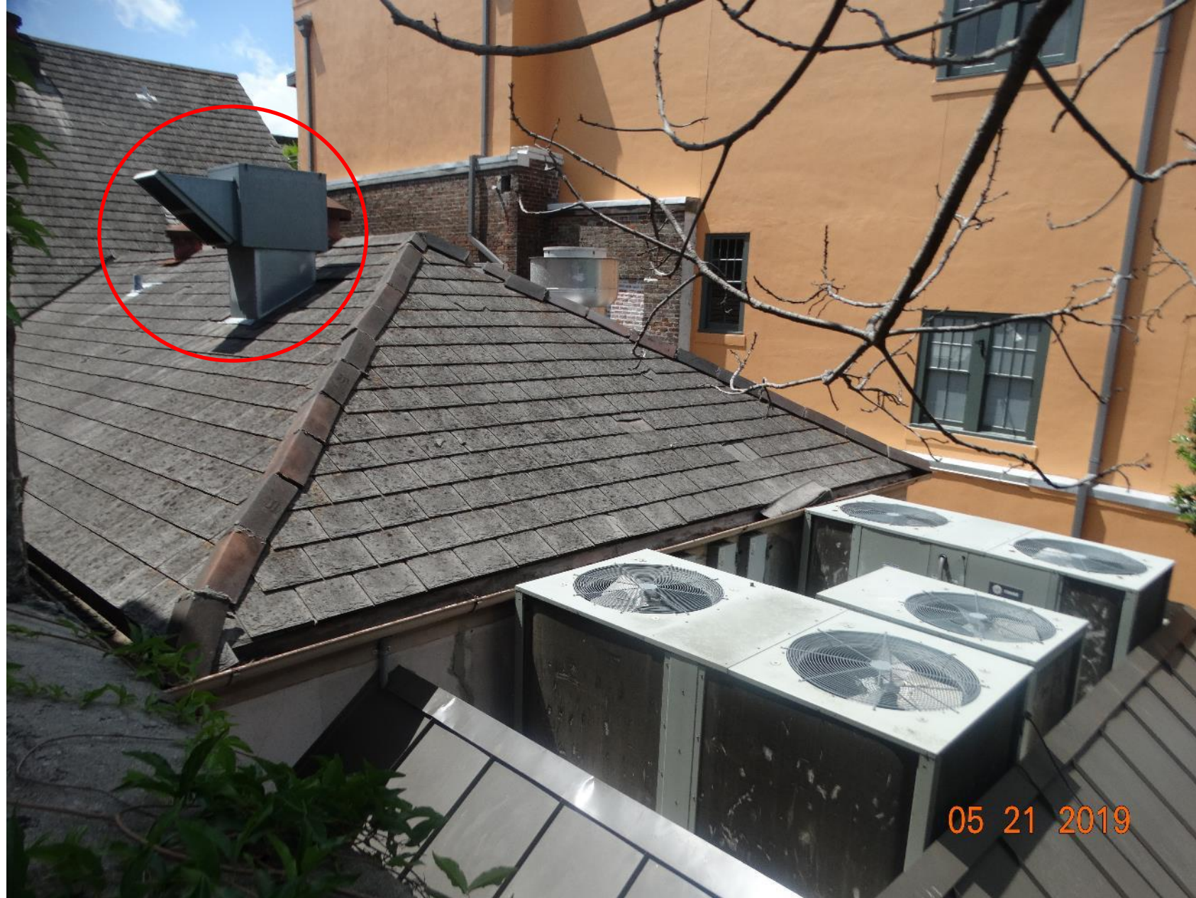
417-19 Bourbon – Previously Existing Air Intake
