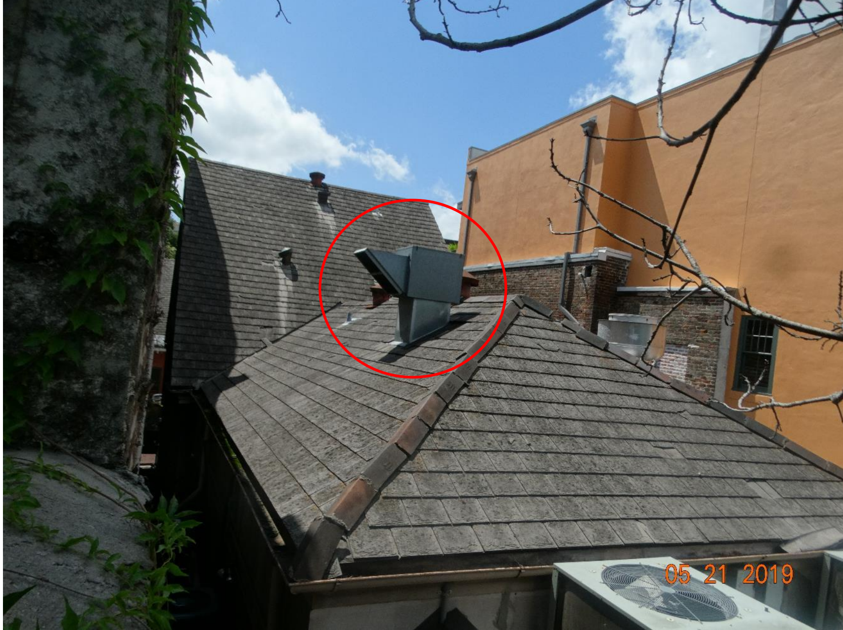
417-19 Bourbon – Previously Existing Air Intake
