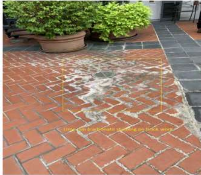
Picture 1916 - Lime salts are present on the surface. Heavy calcium carbonate staining. Pattern of stain shows a poor drainage condition and an area of ponding water.
