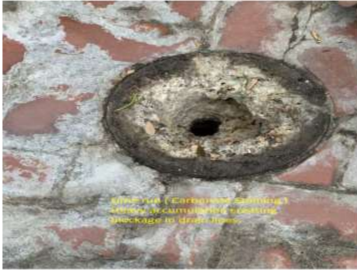
Picture 1915 - Lime run (Carbonate Staining). Heavy accumulation around drain hub impeding the flow of water through the drain line.
