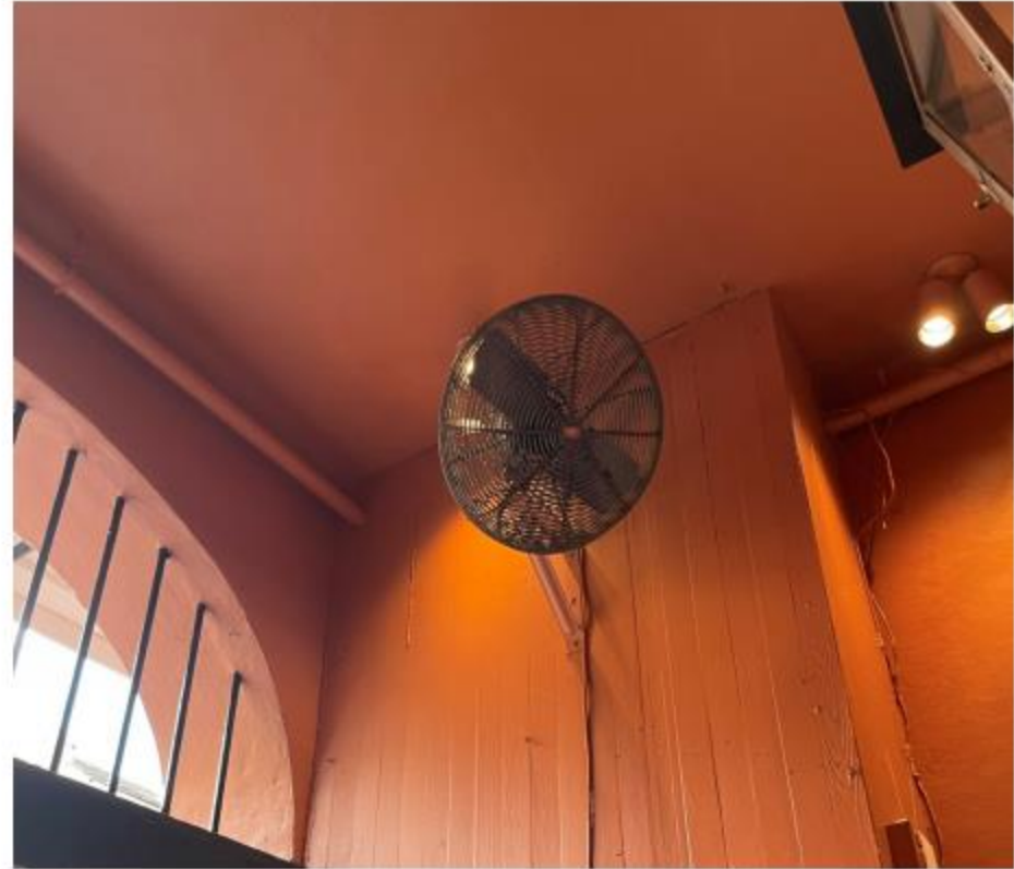
EXISTING WALL MOUNT FAN AT ENTRY
