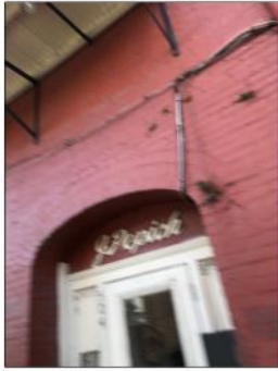
A) DUMAINE STREET [8][14] VEGETATION / WIRING / CONDUIT
