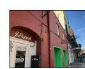
K) DUMAINE STREET [14][8] VEGETATION / WIRING / CONDUIT
