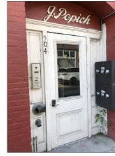
D) DUMAINE STREET [5][8][14] WIRING / DOOR HARDWARE / VEGETATION
