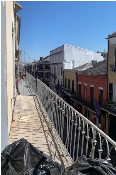
3RD FLOOR BALCONY EXISTING RAILING- APPROX. 2" OFF DECK PROPOSING NEW HORIZONTAL BAR TO SIT 2" FROM BOTTOM OF DECK
