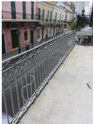
3RD FLOOR BALCONY EXISTING RAILING- SAT DIRECTLY ON THE DECK- PROPOSING NEW HORIZONTAL BAR TO SIT 2" FROM BOTTOM OF DECK
