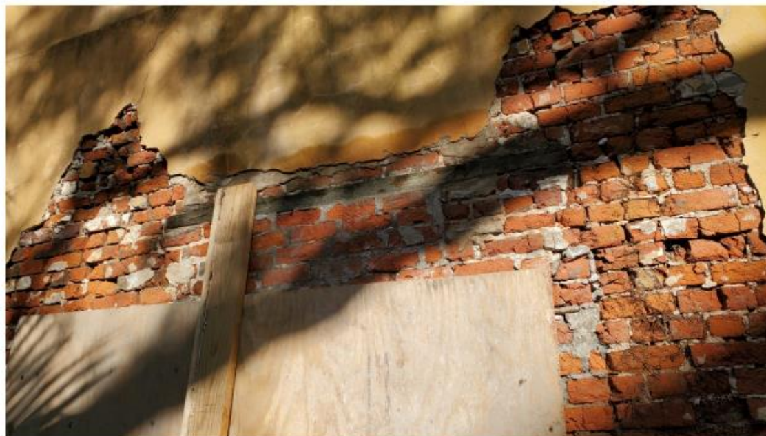
Photo 2: Embedded wood in masonry. bricks in generally poor condition.
