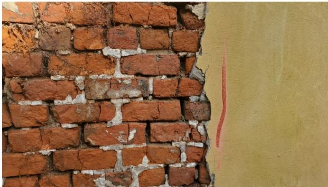
Photo 1: Wall to be repaired, missing mortar cracked, cracked brick.
