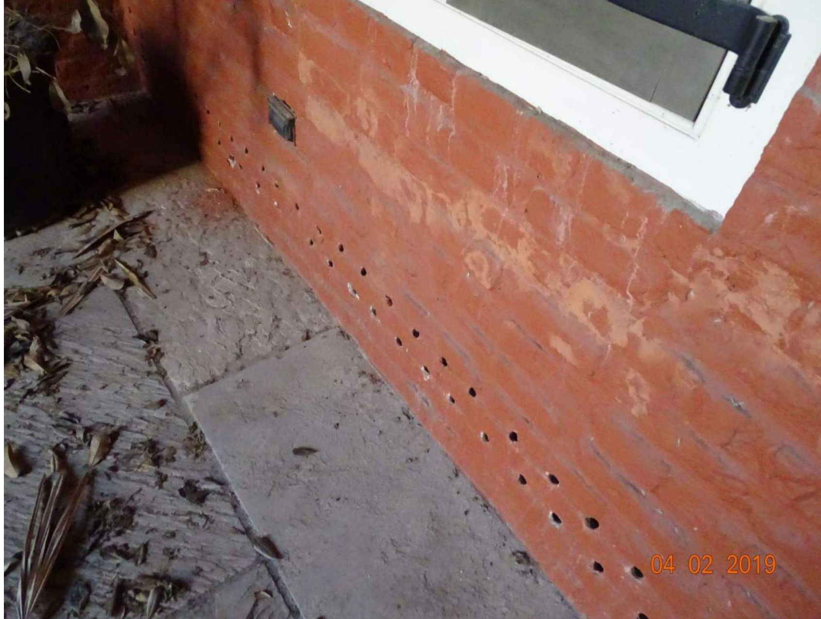
1000 N. Rampart, 1029-35 St. Philip – dampcourse example
