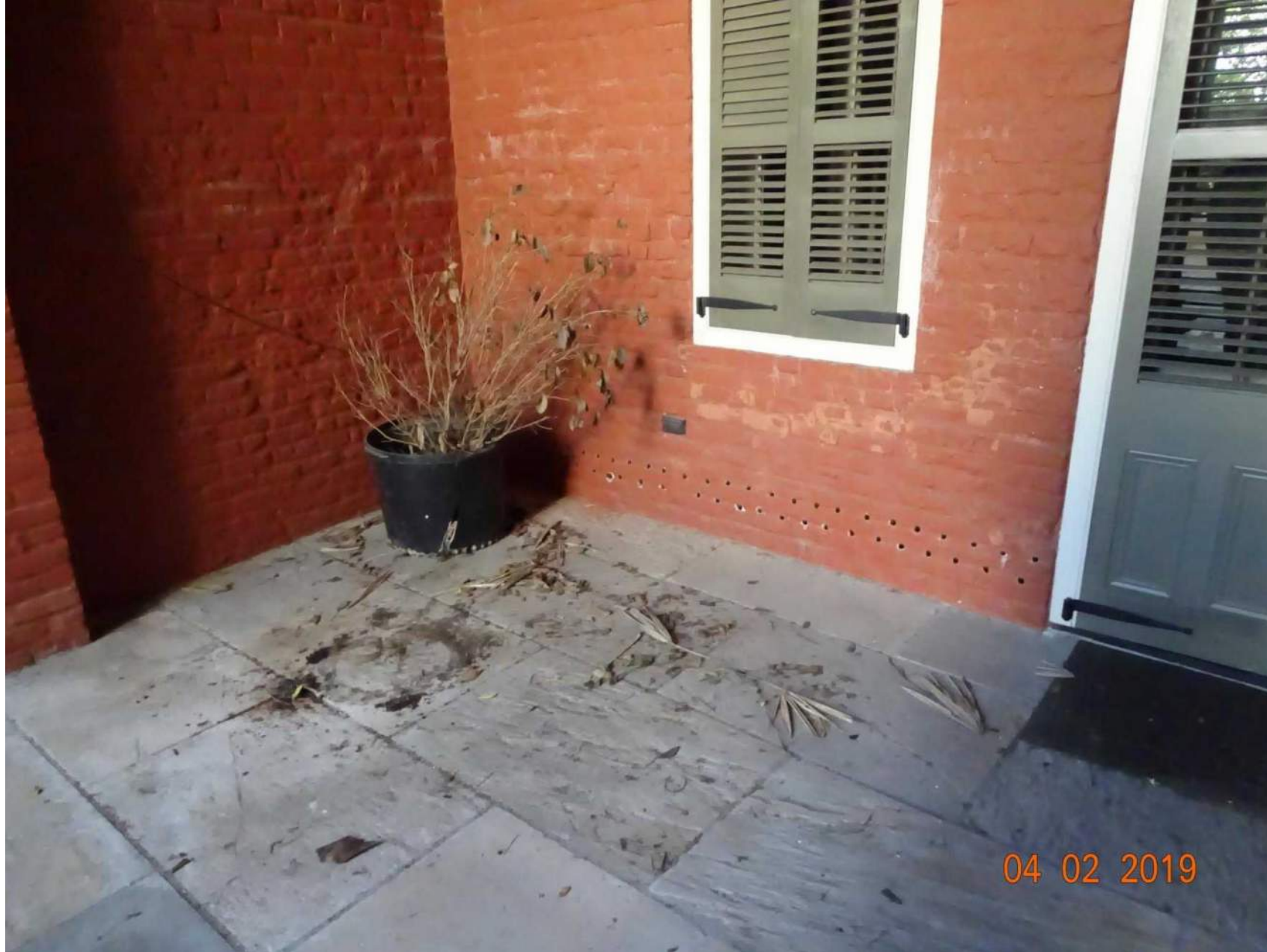
1000 N. Rampart, 1029-35 St. Philip – dampcourse example
