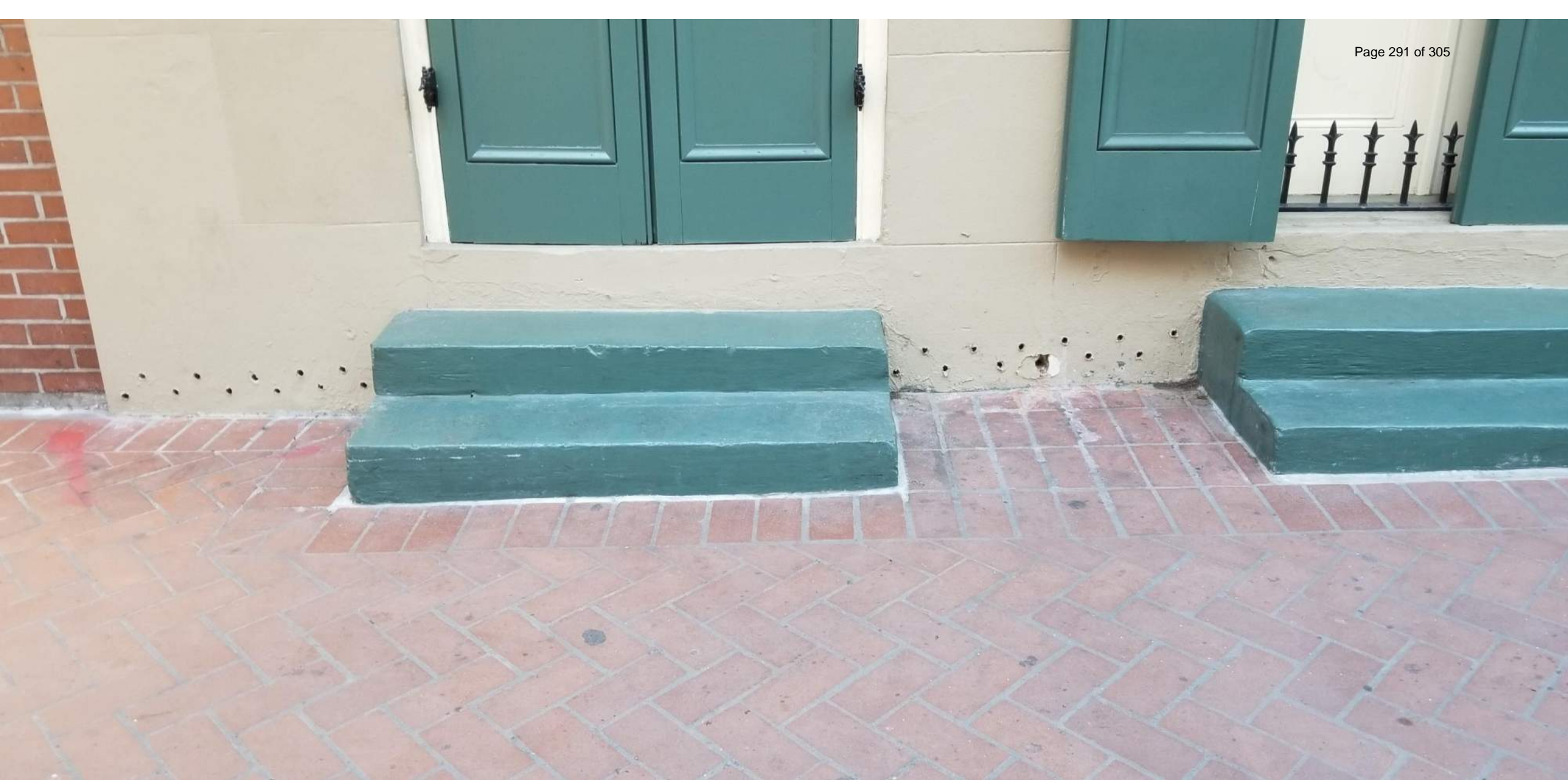
1000 N. Rampart, 1029-35 St. Philip – dampcourse example
