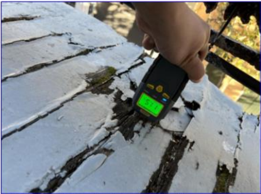
REFERENCE PHOTO OF DAMAGED WOOD. UNIT 10.
