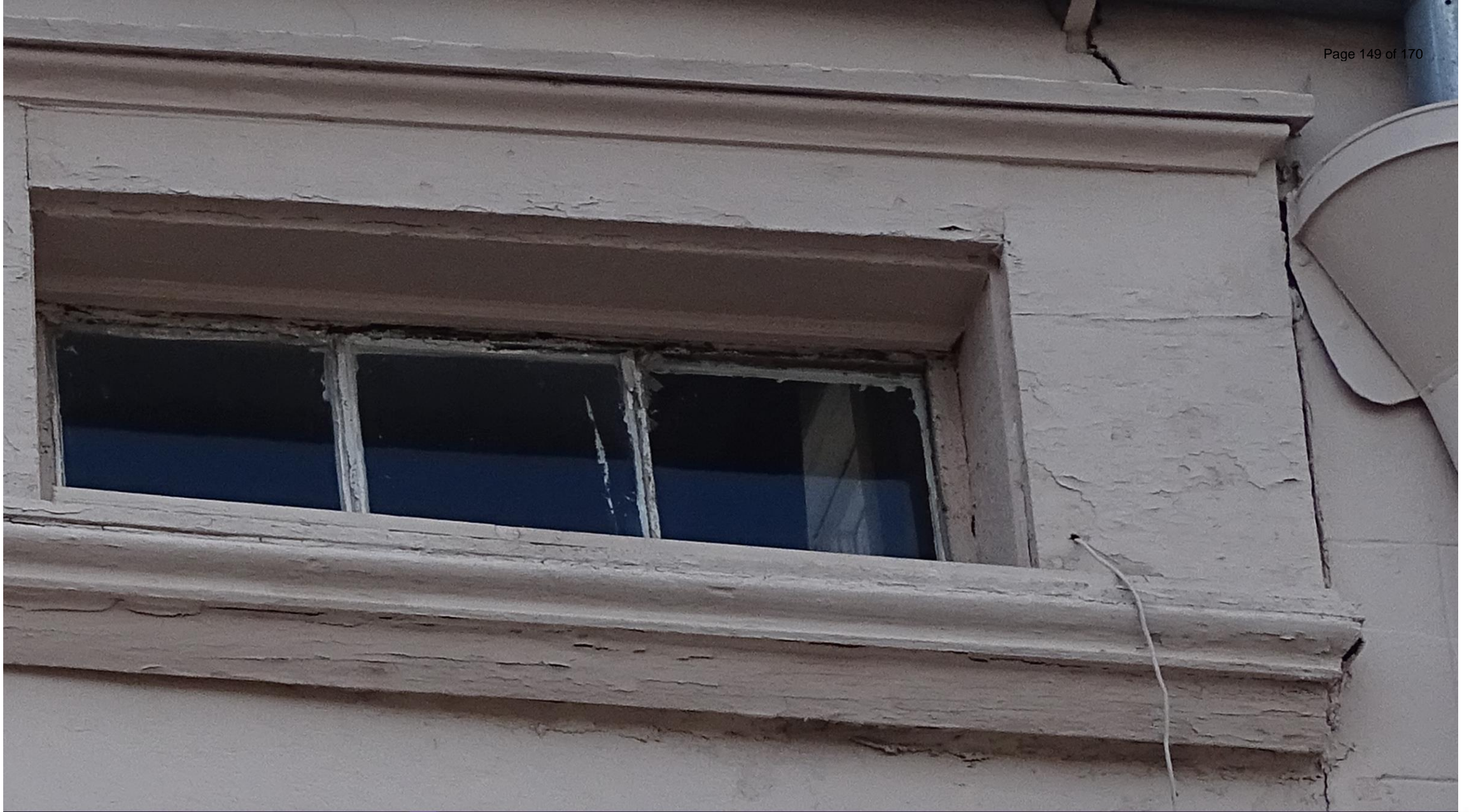
1008 Dauphine – previous band above and below frieze windows
