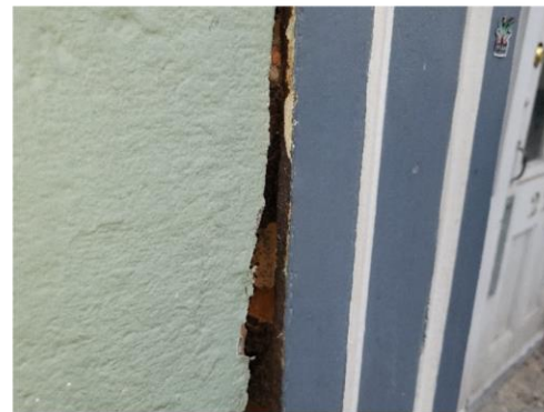
Another close-up view of separation at the side of the left front pilaster
