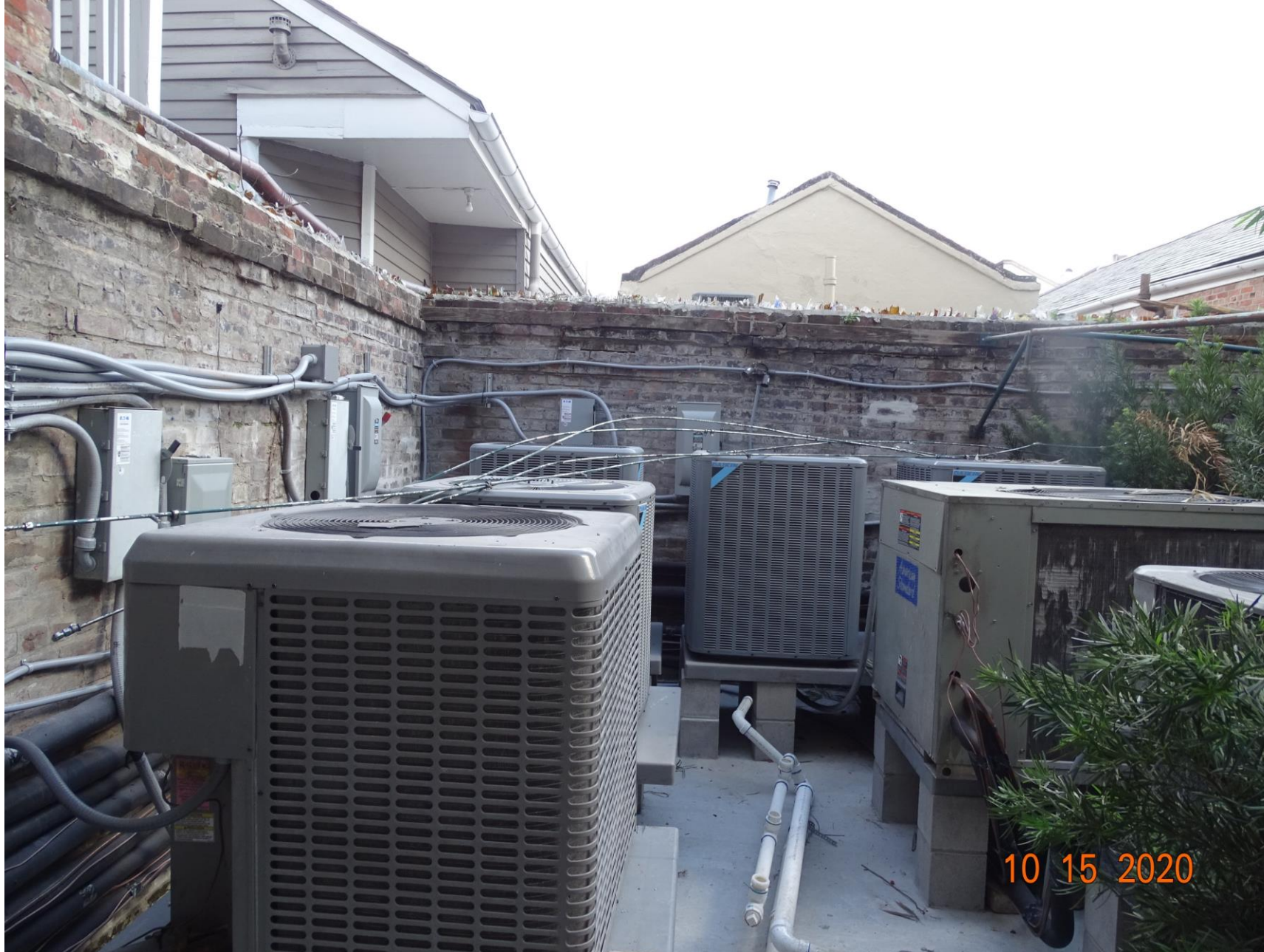
711 Bourbon – Current Mechanical Equipment
