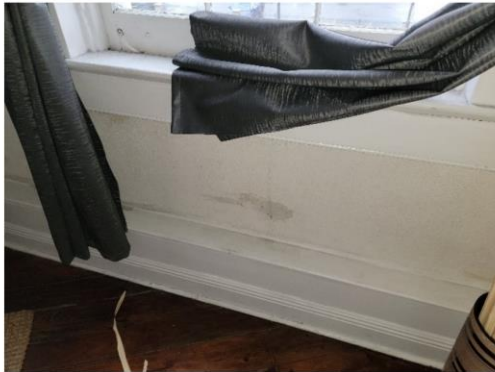
Hairline cracking under the left window on the front wall of Unit No. 1
