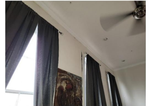
Another view of the separations between the window trim and the front wall in Unit No. 1
