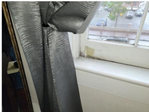
Damaged sash at the right window on the front wall of Unit No. 1
