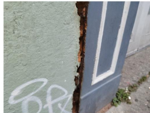
Close-up view of the separation at the side of the left front pilaster
