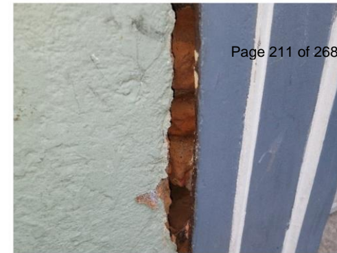
Another close-up view of separation at the side of the left front pilaster
