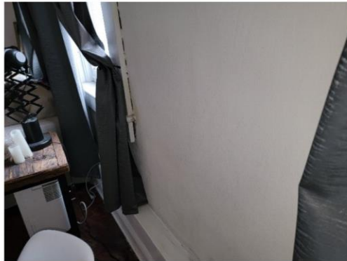
Separation between the trim at the middle windows and the front wall in Unit No. 1
