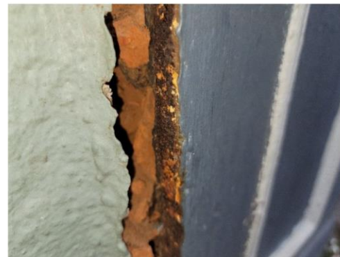
Another close-up view of the side of the cast iron facing at the left front pilaster
