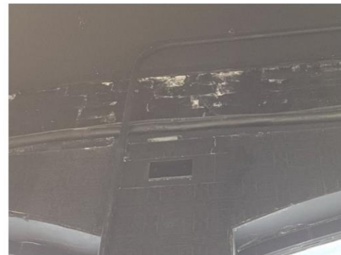
View of the interior of the wall above the middle pilaster on the front wall
