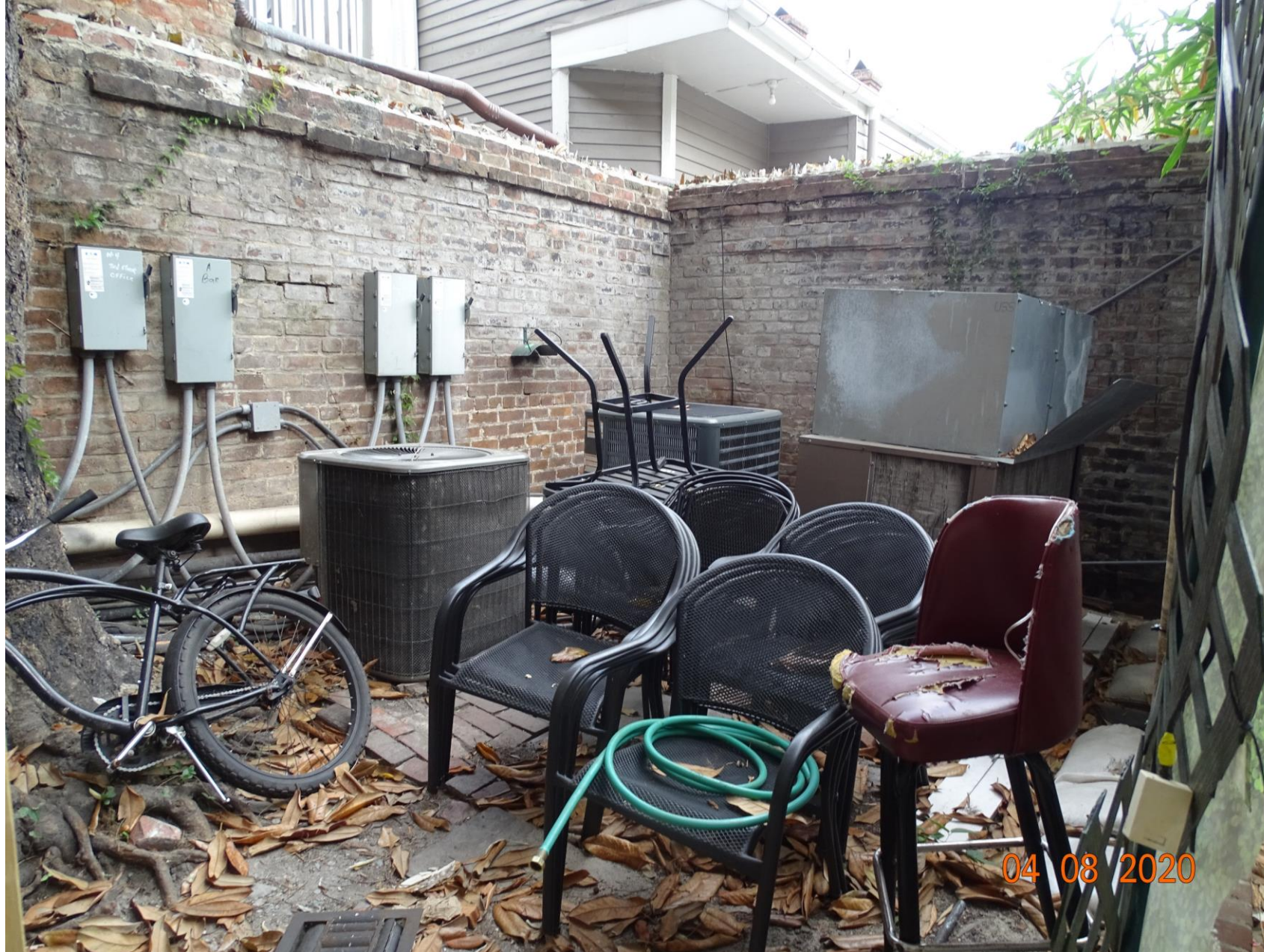
711 Bourbon – Mechanical Equipment April 2020
