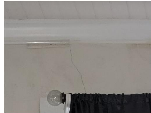
Cracking above the right middle window on the front wall of Unit No. 1
