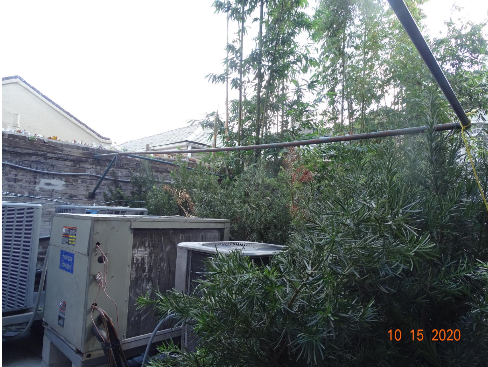
711 Bourbon – Current Mechanical Equipment
