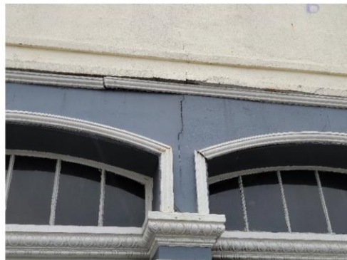
Close-up of the stucco cracking above the middle pilaster on the front wall
