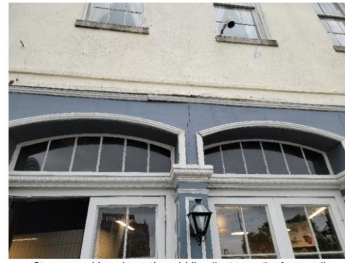
Stucco cracking above the middle pilaster on the front wall
