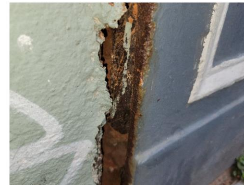
Another close-up view of the side of the cast iron facing at the left front pilaster
