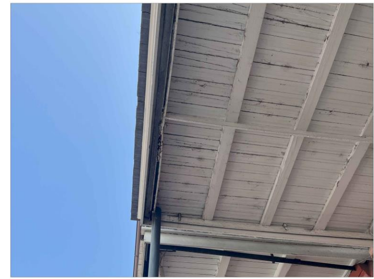
PHOTOGRAPH FROM BELOW SHOWING EXISTING CONDITIONS OF BALCONY
