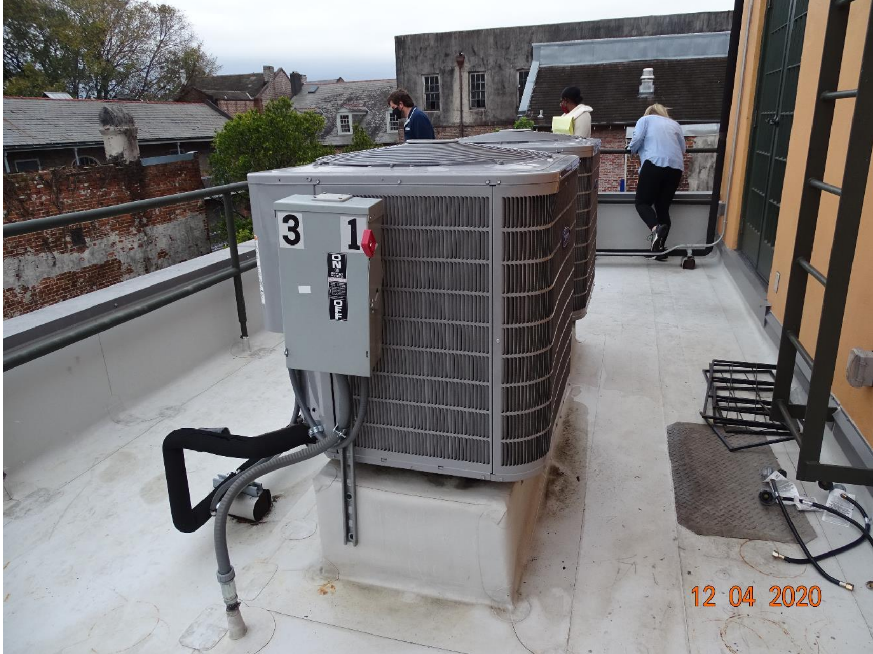
411 Bourbon – Mechanical Equipment – Main Building – As-Built – Third Floor Roof
