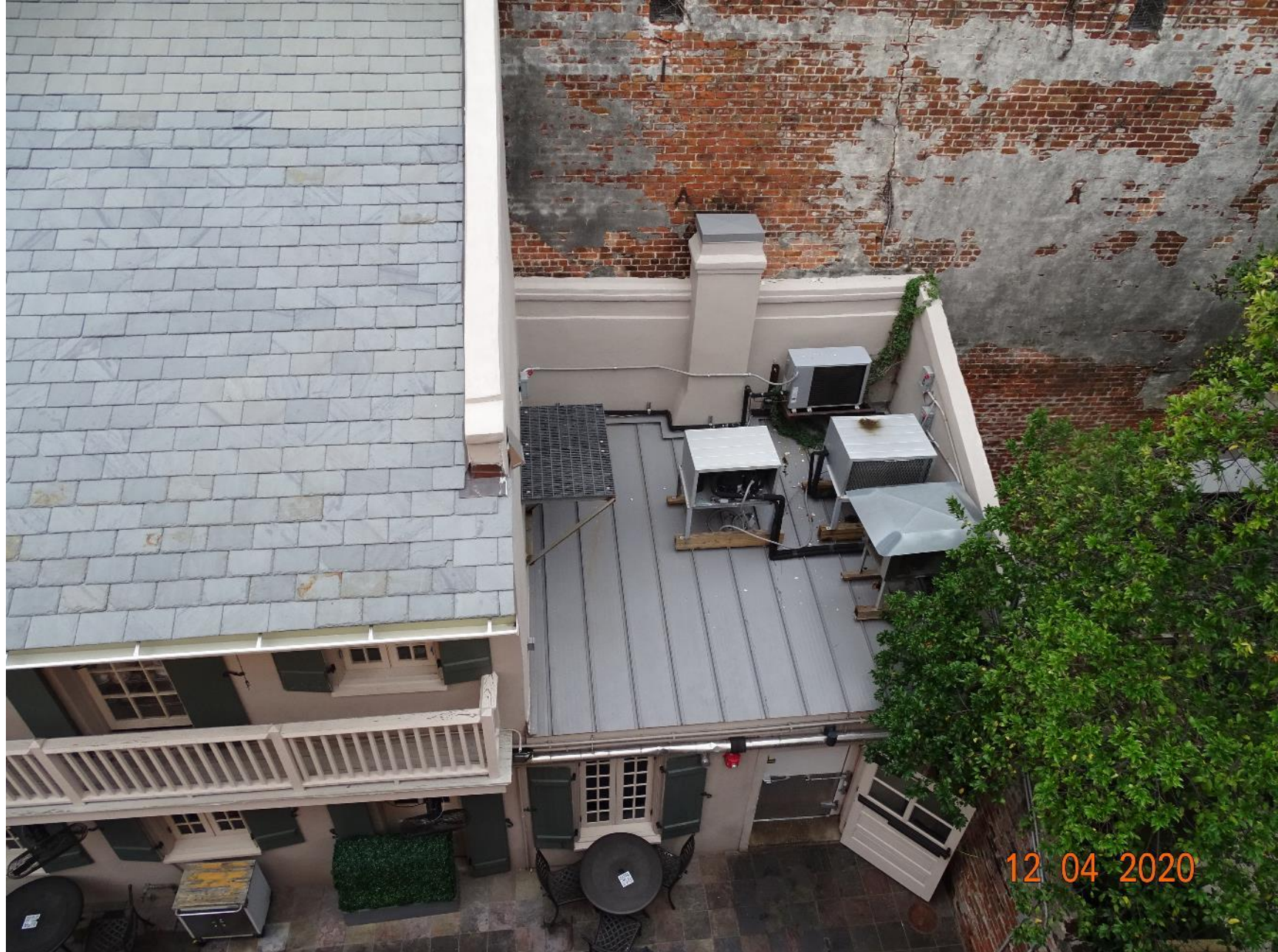
411 Bourbon – Mechanical Equipment – Rear Building – As Built
