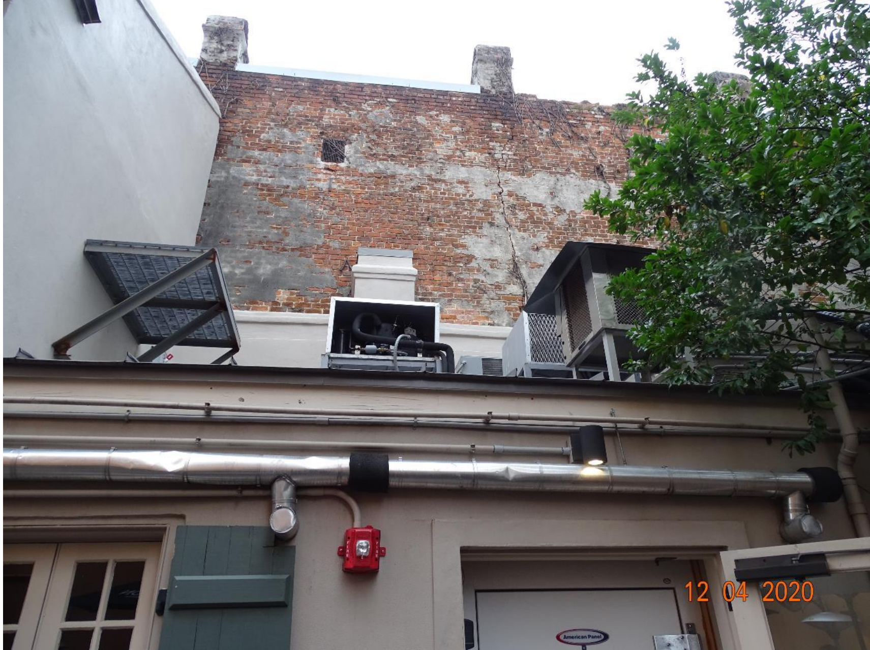
411 Bourbon – Mechanical Equipment – Rear Building – As Built
