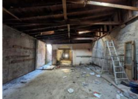
Courtyard roof to be demolished. Slab to be leveled and prepared for pavers
