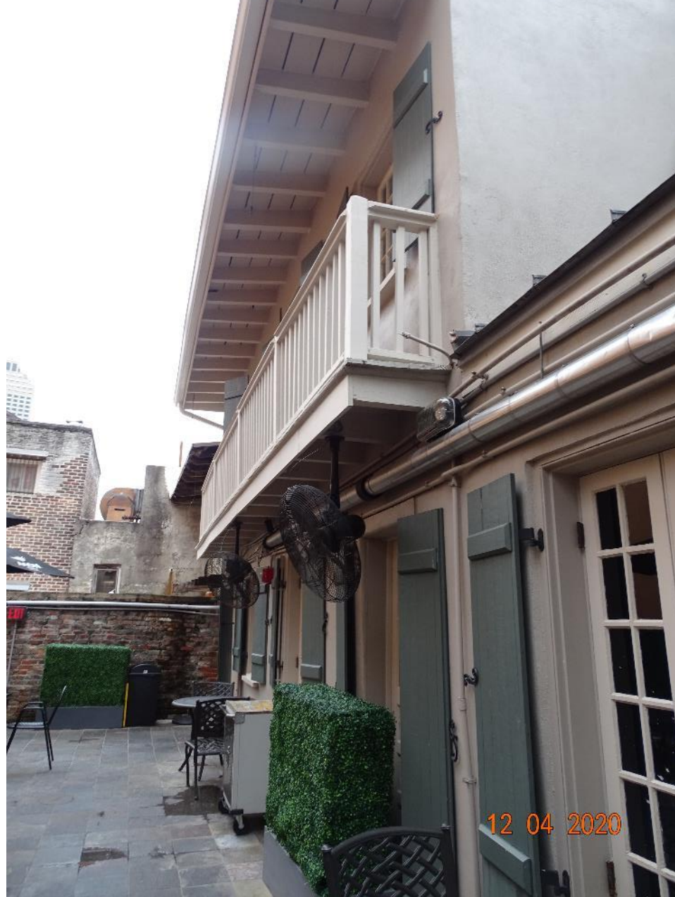
411 Bourbon – Exterior Conduit/Ducting – Rear Building – As Built
