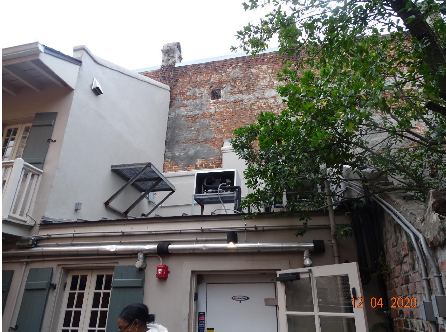
411 Bourbon – Mechanical Equipment – Rear Building – As Built
