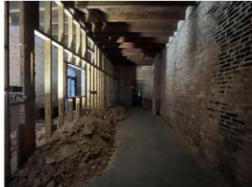
Center stud wall to be removed. Floor to be demoed as needed to provide new footings along columns
