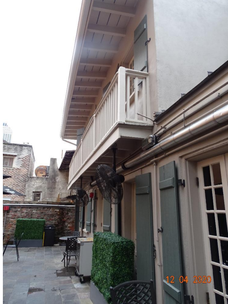
411 Bourbon – Mechanical Equipment – Rear Building – As Built
