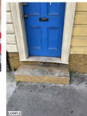
REPAIR AND REWELL AS NECESSARY ALL DAMAGED DOOR MILLWORK
