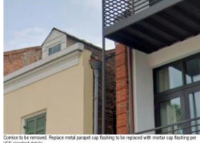
Cornice to be removed. Replace metal parapet cap flashing to be replaced with mortar cap flashing per VCC standard details
