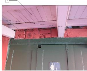
9 BRICK DAMAGE AT SERVANT QUARTER BLDG SCALE: NOT TO SCALE
