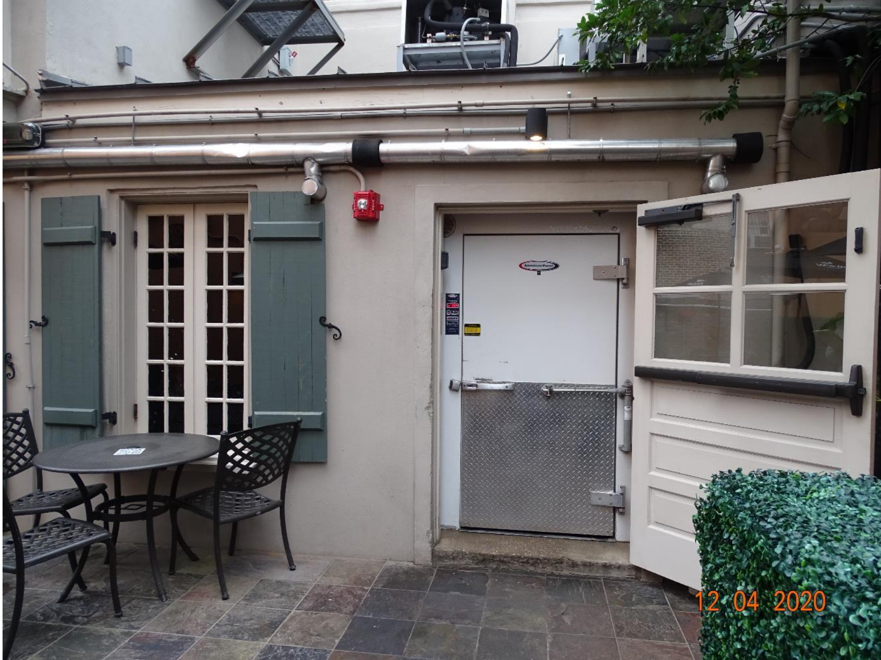
411 Bourbon – Mechanical Equipment – Rear Building – As Built
