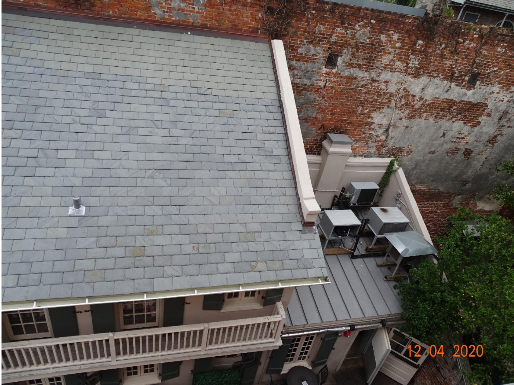
411 Bourbon – Mechanical Equipment – Rear Building – As Built
