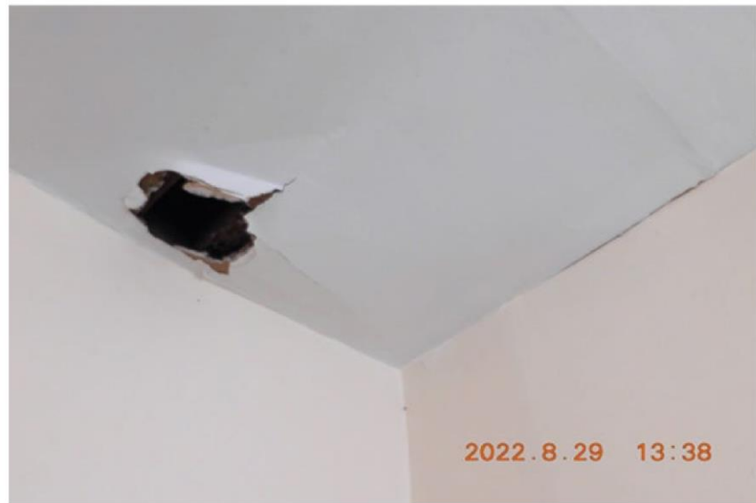
Puncture and Water damage at Second Floor Unit
