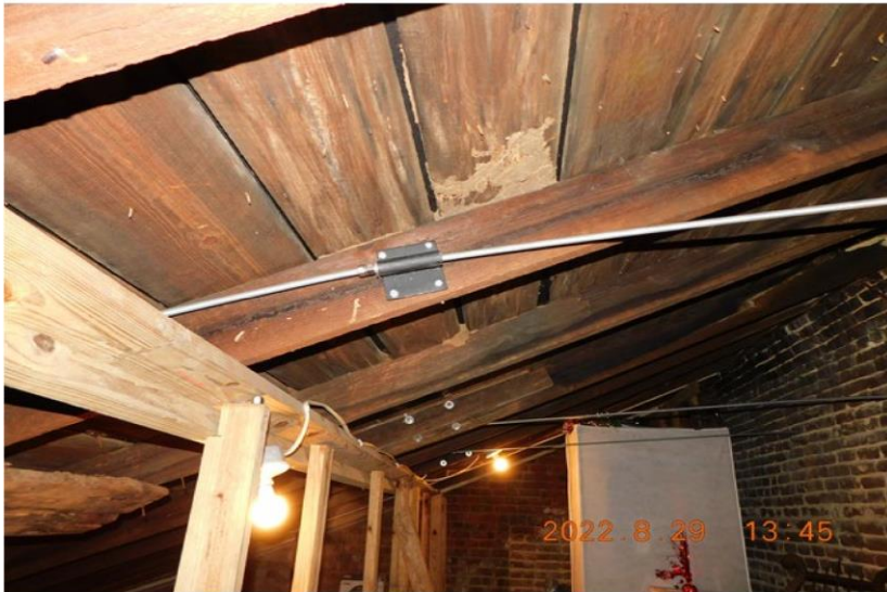
Typical Condition of Brick Tie Rods
