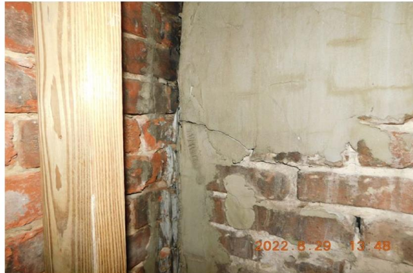
Cracks and Separation at Grout Repair
