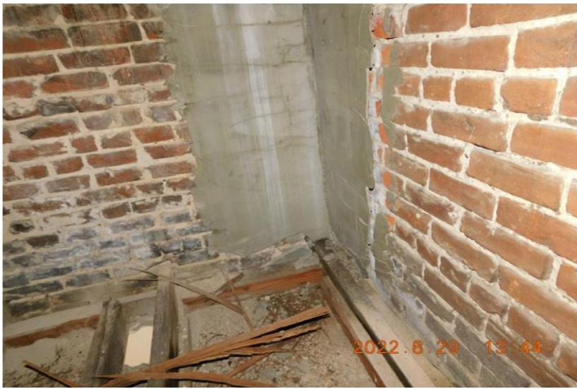
Cracks and Water Damage to Grout repair
