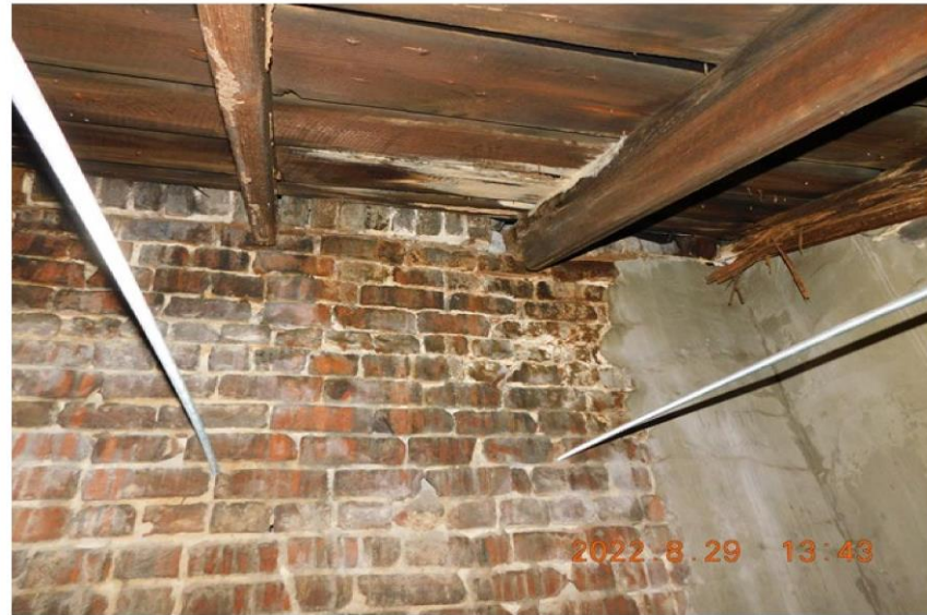
Missing Brick at Roof above Puncture
