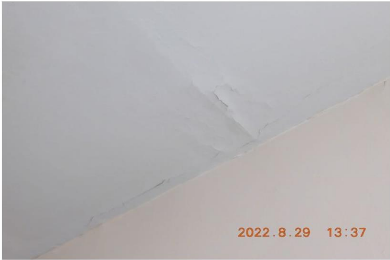
Water Damage and Cracks at Second Floor Unit
