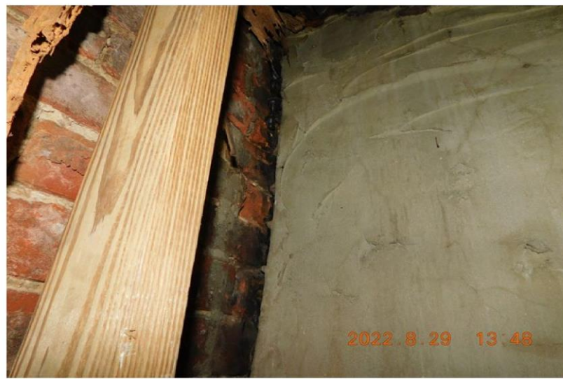
Signs of Movement at Grout Repair
