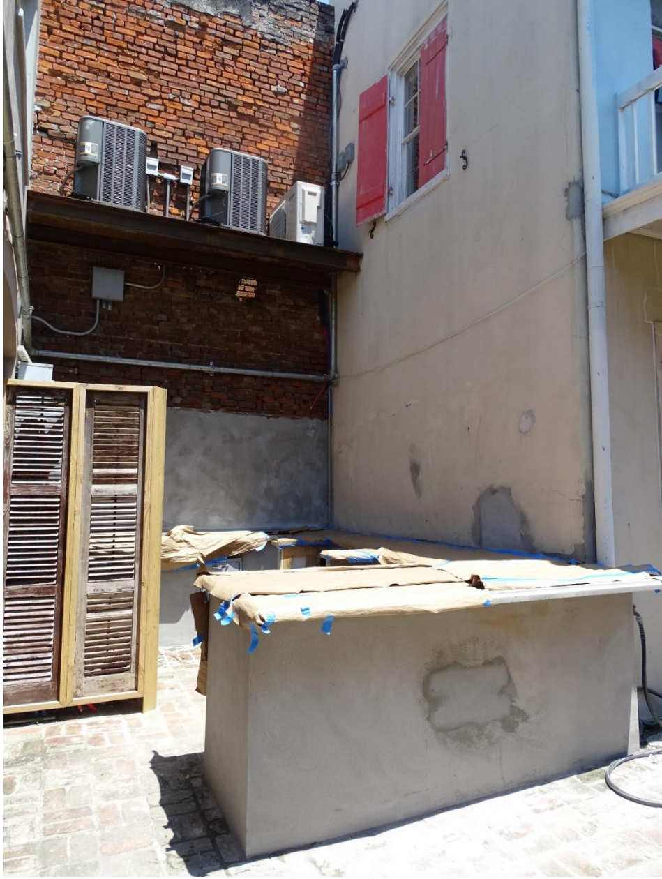
1118 Burgundy – unpermitted exterior kitchen
