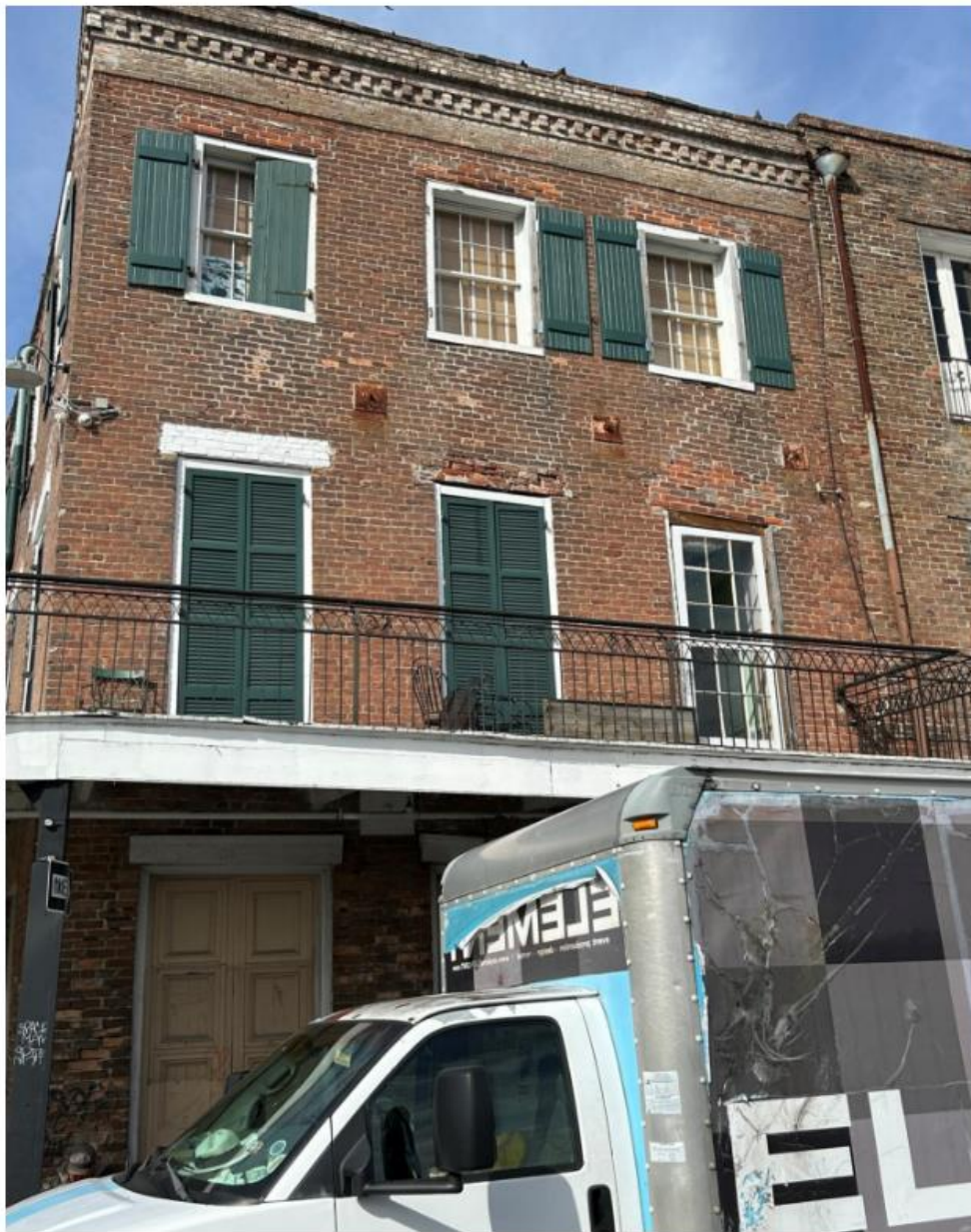
EAST SIDE BUILDING – LINTELS TO BE REPLACED
