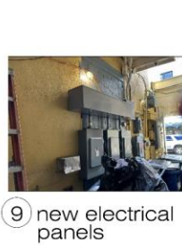
9 new electrical panels
