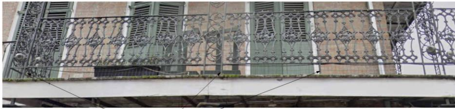
VERTICAL SUPPORT, ALIGN NEW GUARDRAIL VERTICAL SUPPORT IN-LINE, TYP. RAILING AT ROYAL, CORNER, AND PART OF ST ANN ST.
