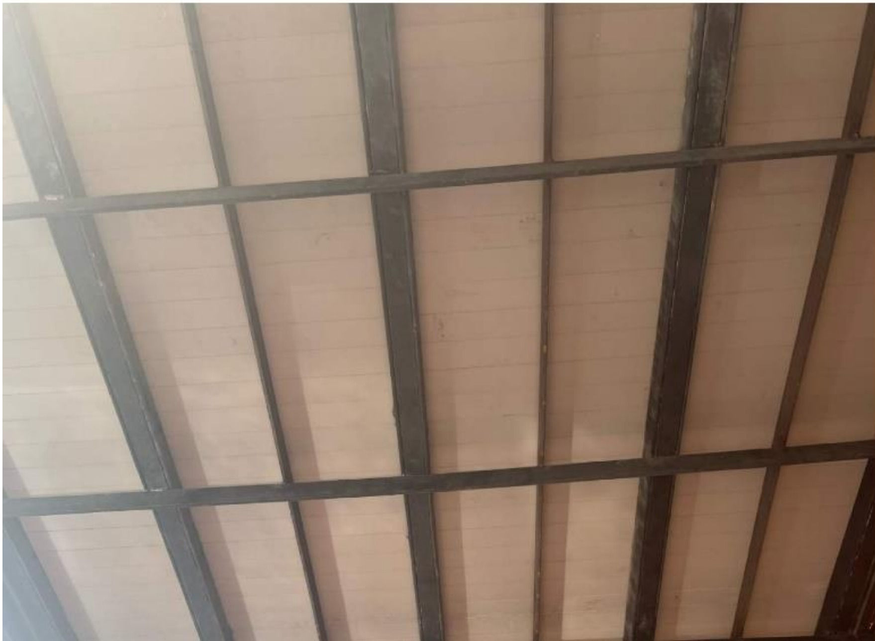
1218 Decatur – Metal support example (incorrectly painted black)
