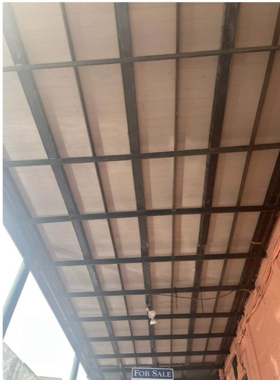
1218 Decatur – Metal support example (incorrectly painted black)
