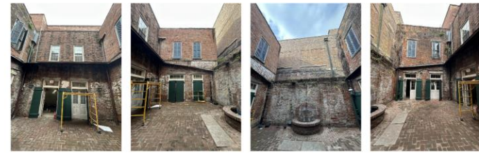
EXISTING CONDITION BLDG ELEVATION - CTYD 1 EXISTING CONDITION BLDG ELEVATION - CTYD 2 EXISTING CONDITION BLDG ELEVATION - CTYD 3 EXISTING CONDITION BLDG ELEVATION - CTYD 4
