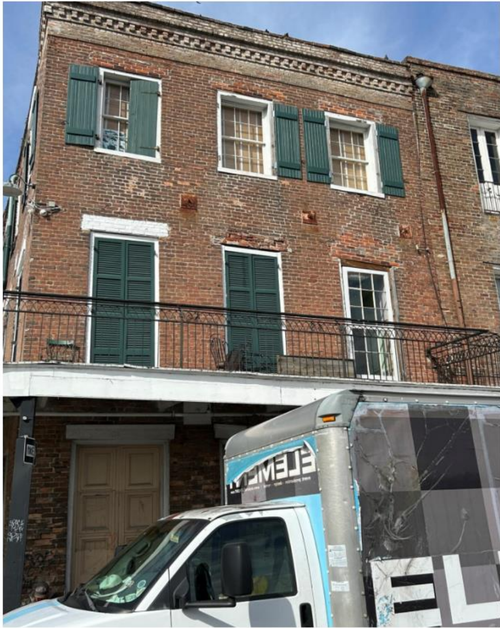
EAST SIDE BUILDING – LINTELS TO BE REPLACED
