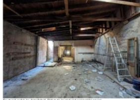
Courtyard roof to be demolished. Slab to be leveled and prepped for pavers.
