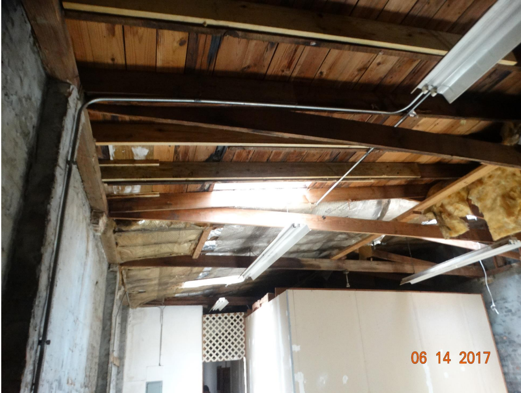
622 N Rampart – in brown-rated portion of building
