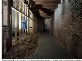
Corner stud wall to be removed. Floor to be demised as needed to provide new footings along exterior.
