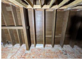
Beams to be demolished per plans. GC to provide all necessary temporary bracing
