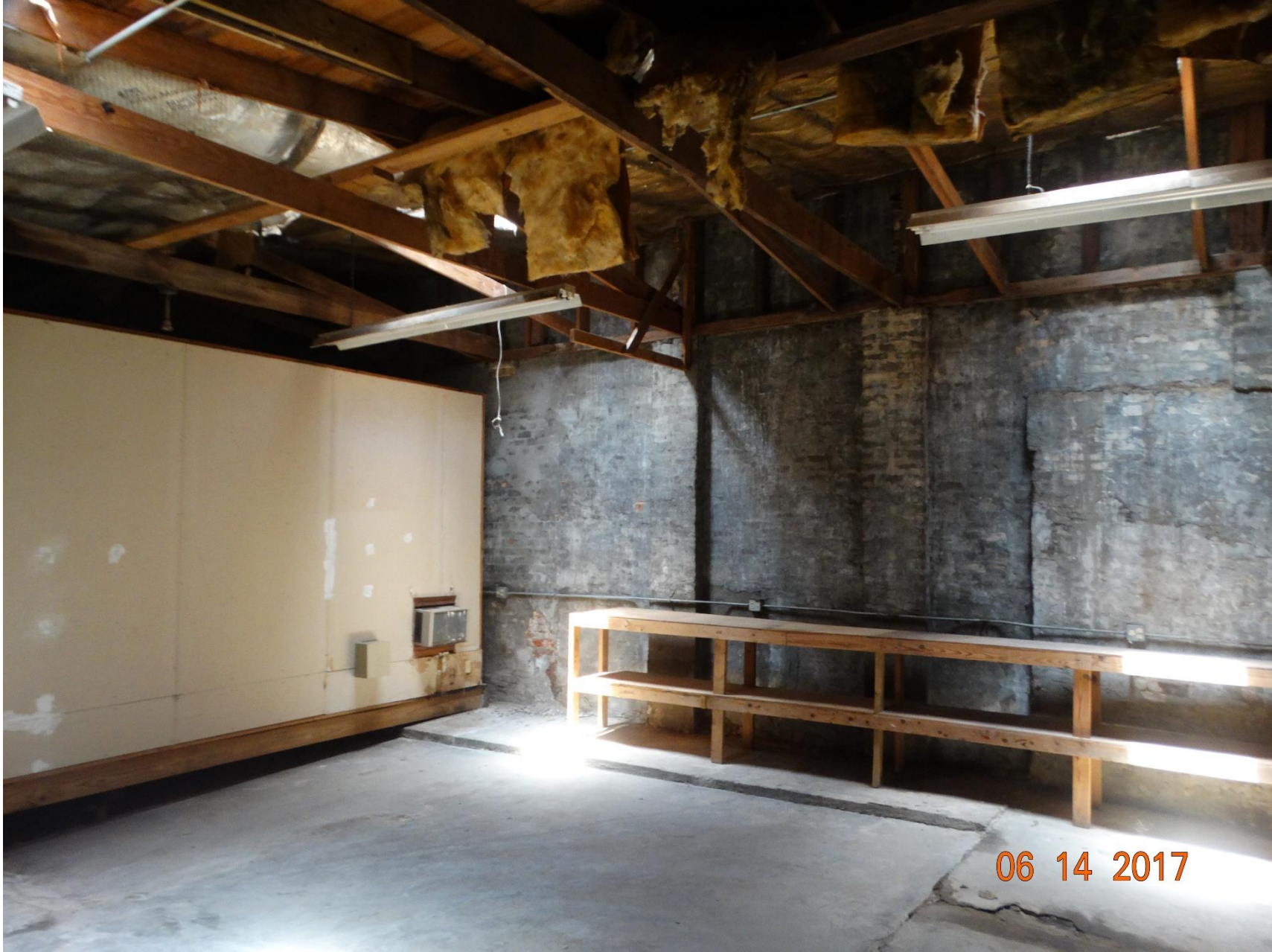
622 N Rampart – in brown-rated portion of building
