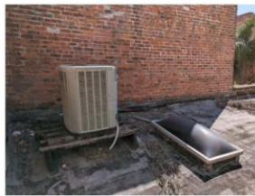
Existing condenser on roof. Roof to be demolished, condenser to be relocated
