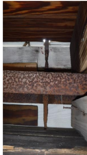
Photo 4: Side of balcony, rust lattice columns.
