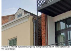
Cornice to be removed. Replace metal parapet cap flashing to be replaced with metal cap flashing per VCC standard details
