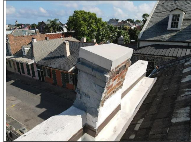
Photograph 5: West side, facing north, brick chimney protrusion.
