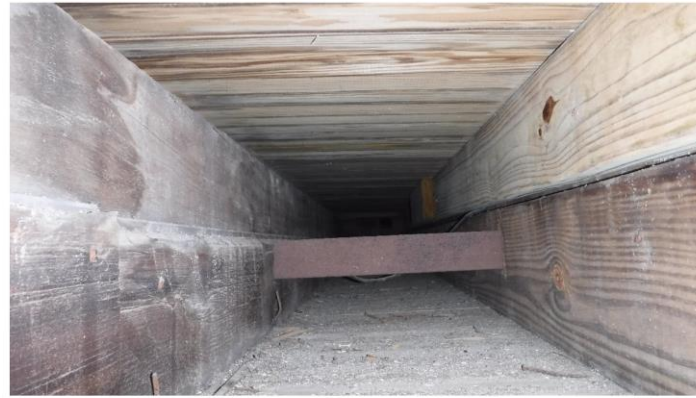
Photo 3: View thru the wood joist, steel support bar can be seen.
