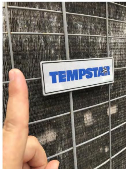
Condenser #1_No tag visible
