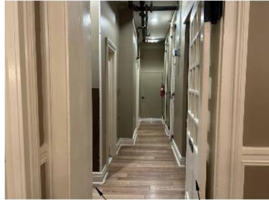
^K EXIT CORRIDOR, EXIT SIGNAGE TO BE ADDED. DEMO DOOR
