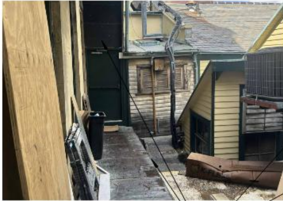
^J LOCATION OF NEW METAL RAIL AND NEW EXIT SIGN.
