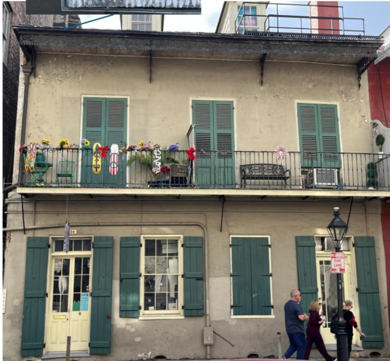
Replace corrugated metal roof and box gutters of balcony awning to match existing.
