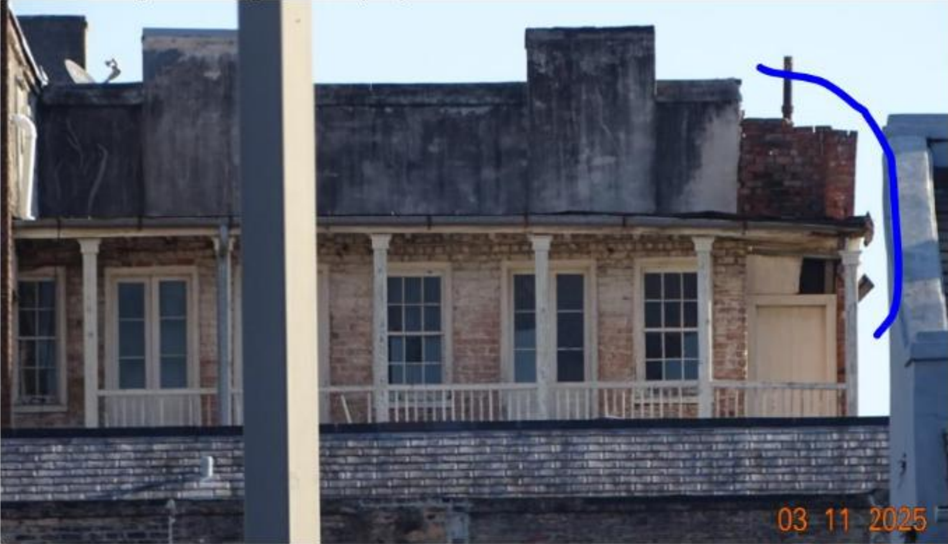
Additional images of bowing section of parapet wall:
