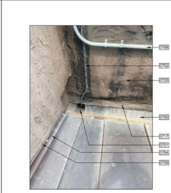
30 CHILLER ROOF - NW GUTTER CORNER
