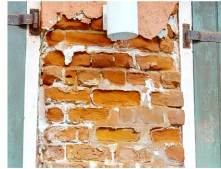
726 TOULOUSE ST - DEPENDENCY BRICK DETERIORATION
