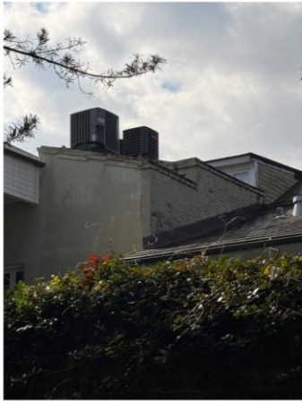
617 DAUPHINE STREET EXISTING ROOFTOP MECHANICAL EQUIPMENT
