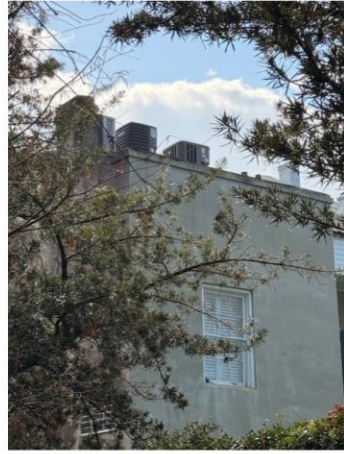
617 DAUPHINE STREET EXISTING ROOFTOP MECHANICAL EQUIPMENT
