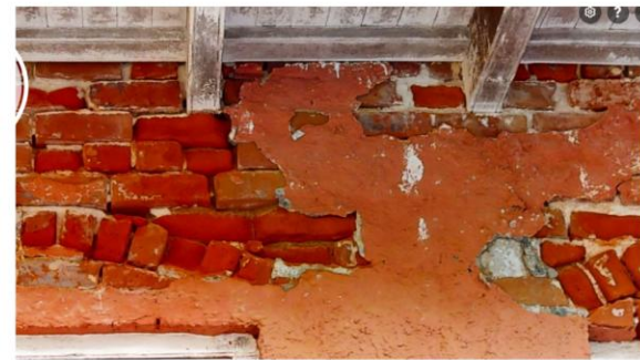
726 TOULOUSE ST - DEPENDENCY BRICK DETERIORATION
