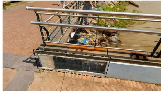
15 EXISTING SITE WALL TO BE REPAIRED 12" x 1'-0"
