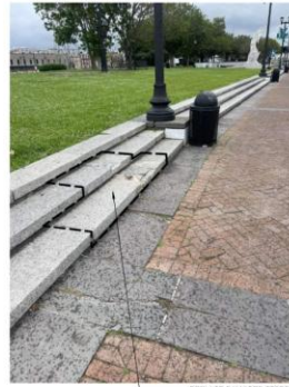
14 EXISTING DAMAGED STEPS 15" x 12" x 1'-0"
