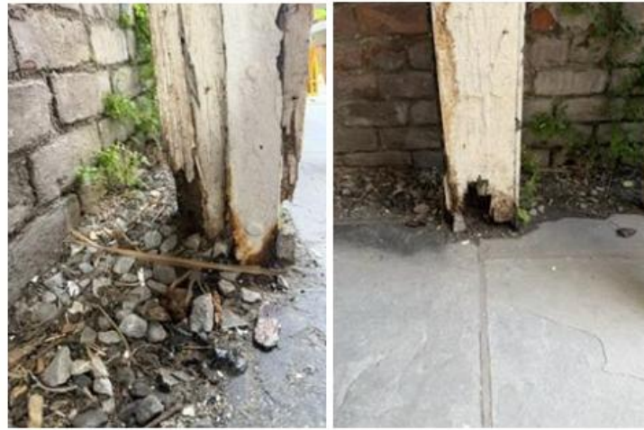
Figure 3.4.3 Damaged posts requiring replacement
