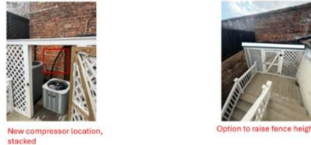
Figure 3.5.2 Details on location of stacked A/C compressor and fence height
