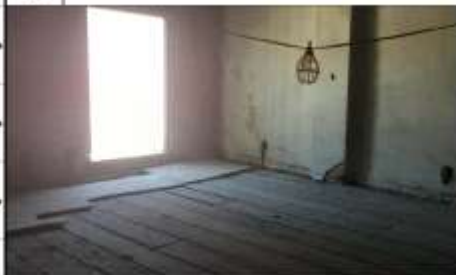
E-1 EXISTING WINDOW CONDITIONS 516 CONTI K73
