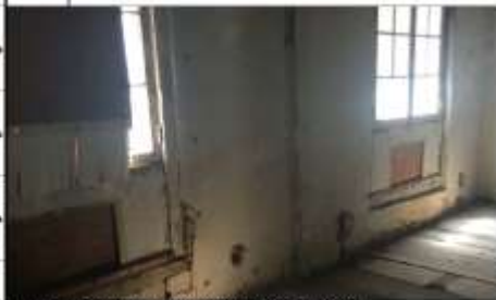
A-1 EXISTING WINDOW CONDITIONS 512 CONTI K73
