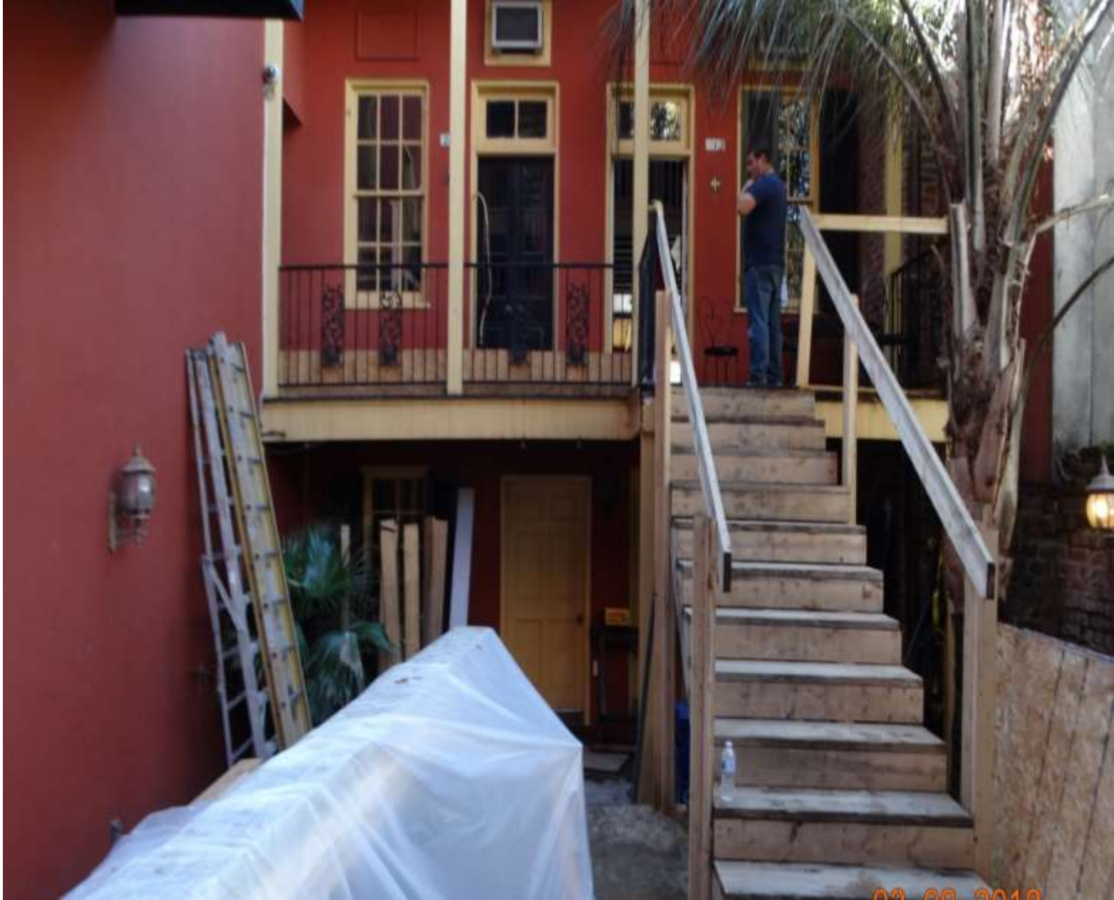
828 Toulouse – Toulouse elevation of 832 rear building
