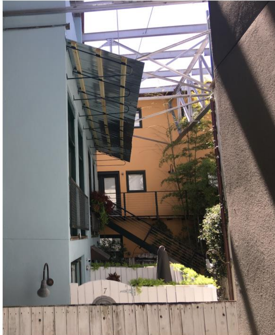
THE AWNING DESIGN BEING APPEALED IS SHOWN ABOVE UNITS 7 and 8. IT EMPLOYS CORRUGATED METAL ON UNPAINTED WOODEN PURLINS ON METAL BRACKETS. THE DESIGN FOCUSES RAINWATER DIRECTLY INTO THE CENTER OF THE PRIVATE PATIO BELOW IT, RATHER THAN OUT-AND-AWAY, OR INTO A CONTROLLED GUTTER AND DOWNSPOUT SYSTEM AS IT COULD.
