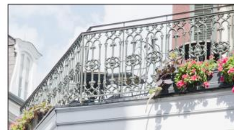
A discrete, higher secondary safety rail has been installed behind the cast iron balustrade to meet building code requirements. An alternative would be to raise the historic balustrade to the required height.
