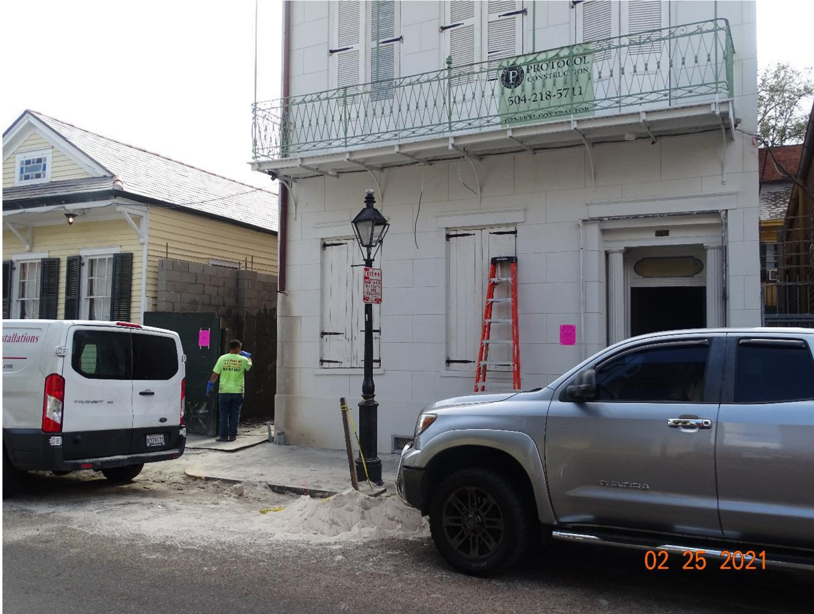
928 St. Ann – 2/25/2021, STOP WORK ORDER PLACED
