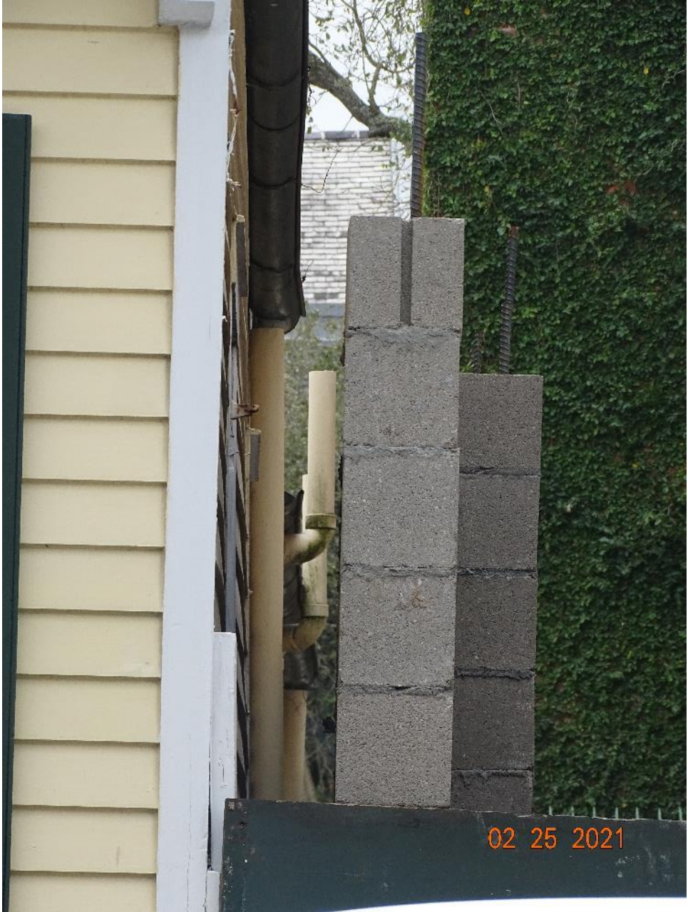
928 St. Ann – 2/25/2021, STOP WORK ORDER PLACED
