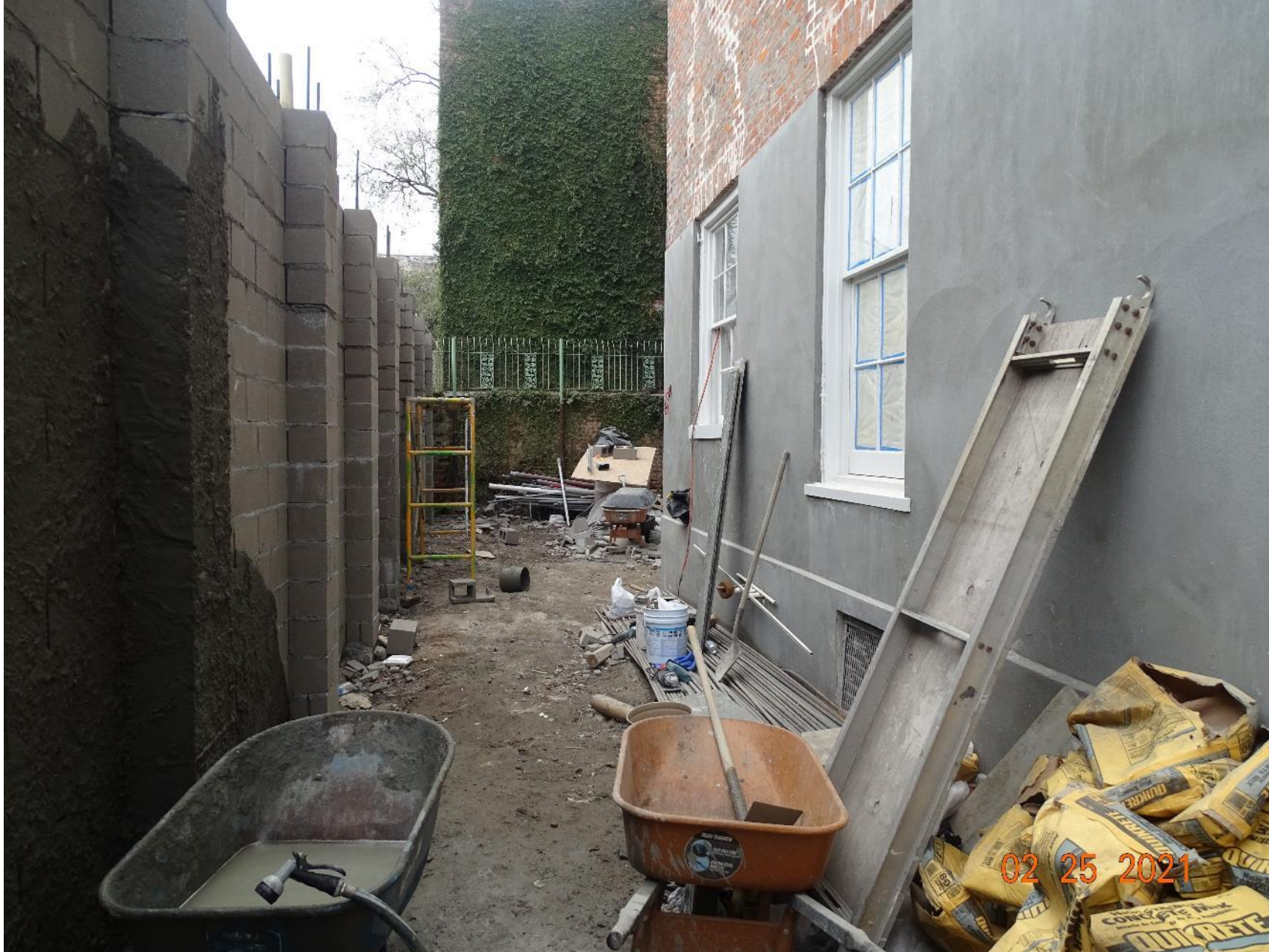
928 St. Ann – 2/25/2021, STOP WORK ORDER PLACED
