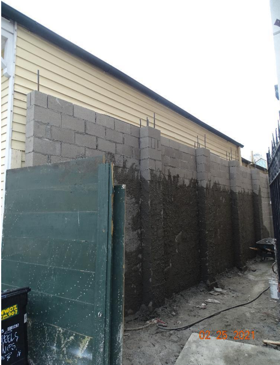
928 St. Ann – 2/25/2021, STOP WORK ORDER PLACED
