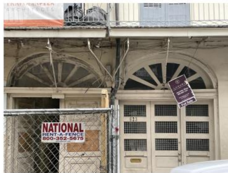
CARRIAGE WAY OPENING SETTLING
