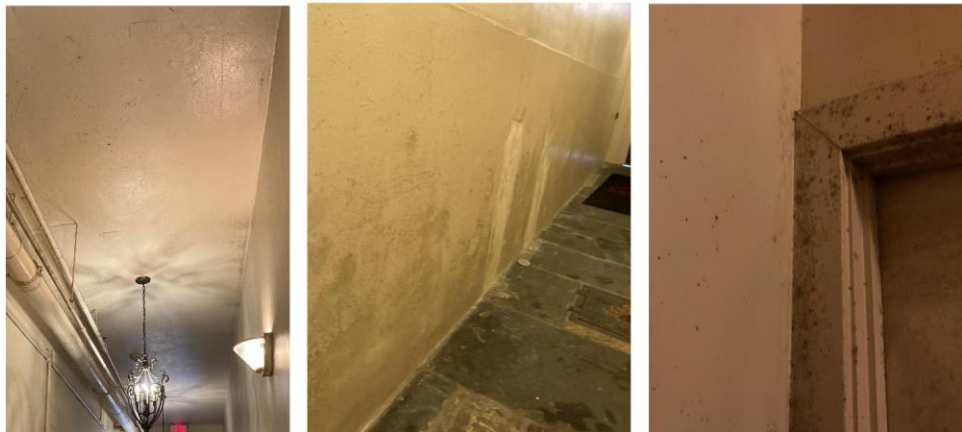
EXISTING MOISTURE DAMAGE WITHIN STAIR CORRIDORS
