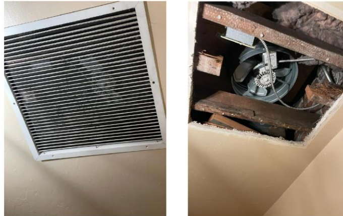
Figure 1: Fans located at grille but not connected
