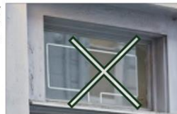
Abandoned security tape on windows should be removed.
