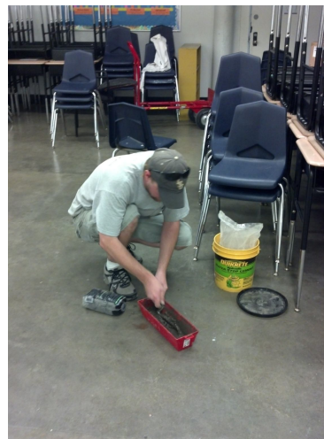
Figure 8. Eric Guidry (Pest Control Inspector 4) prepared the concrete for patching holes at John McDonogh High School.
