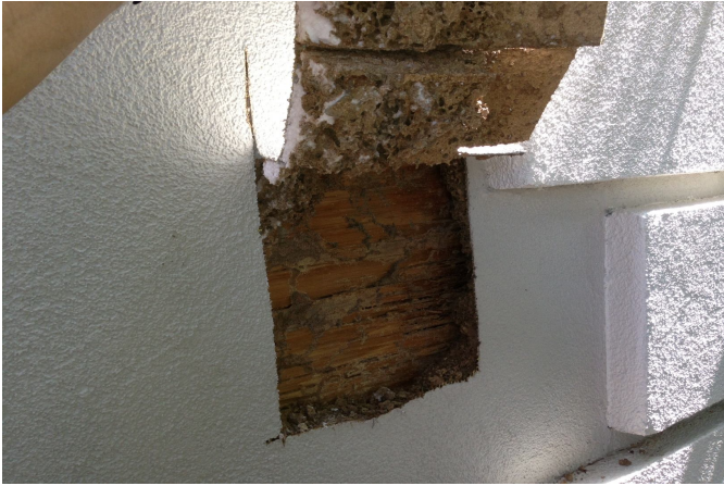
Figure 20. Termite damage to the plywood behind the EIFS. This Formosan termite infestation was caused by a roof flashing issue allowing rain to percolate.
