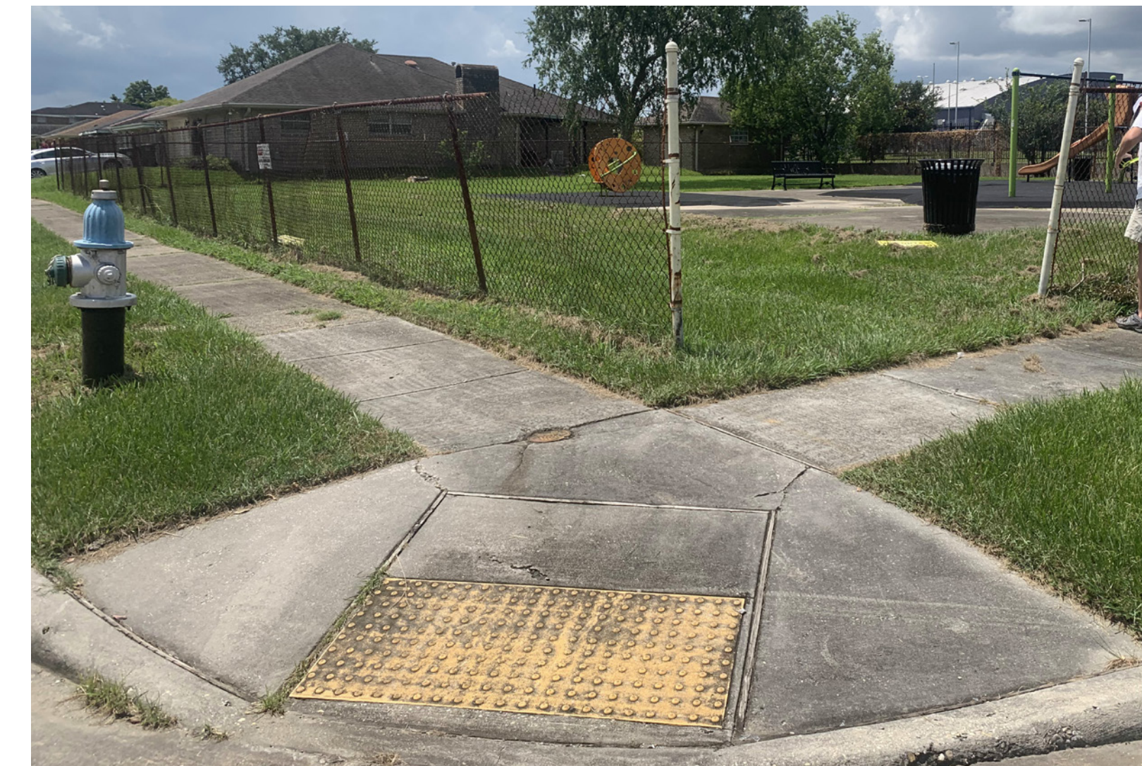
ADA ramp to sidewalk but no ADA access to the play structure.
