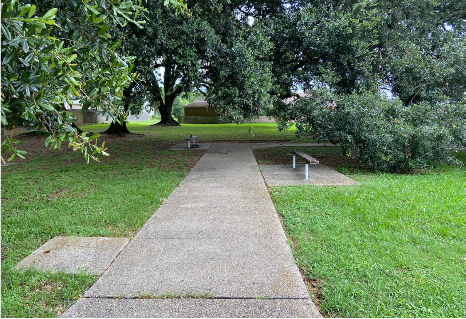
ADA ramp to sidewalk but no ADA access to the play structure.
