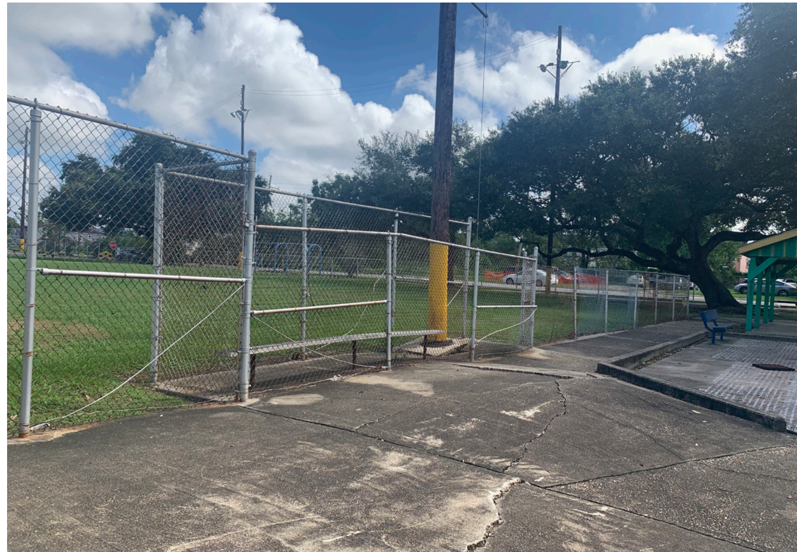
Rusted backstop fence and uneven walkway.
