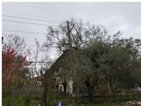
Pole mounted transformer along Vespasian Blvd.
