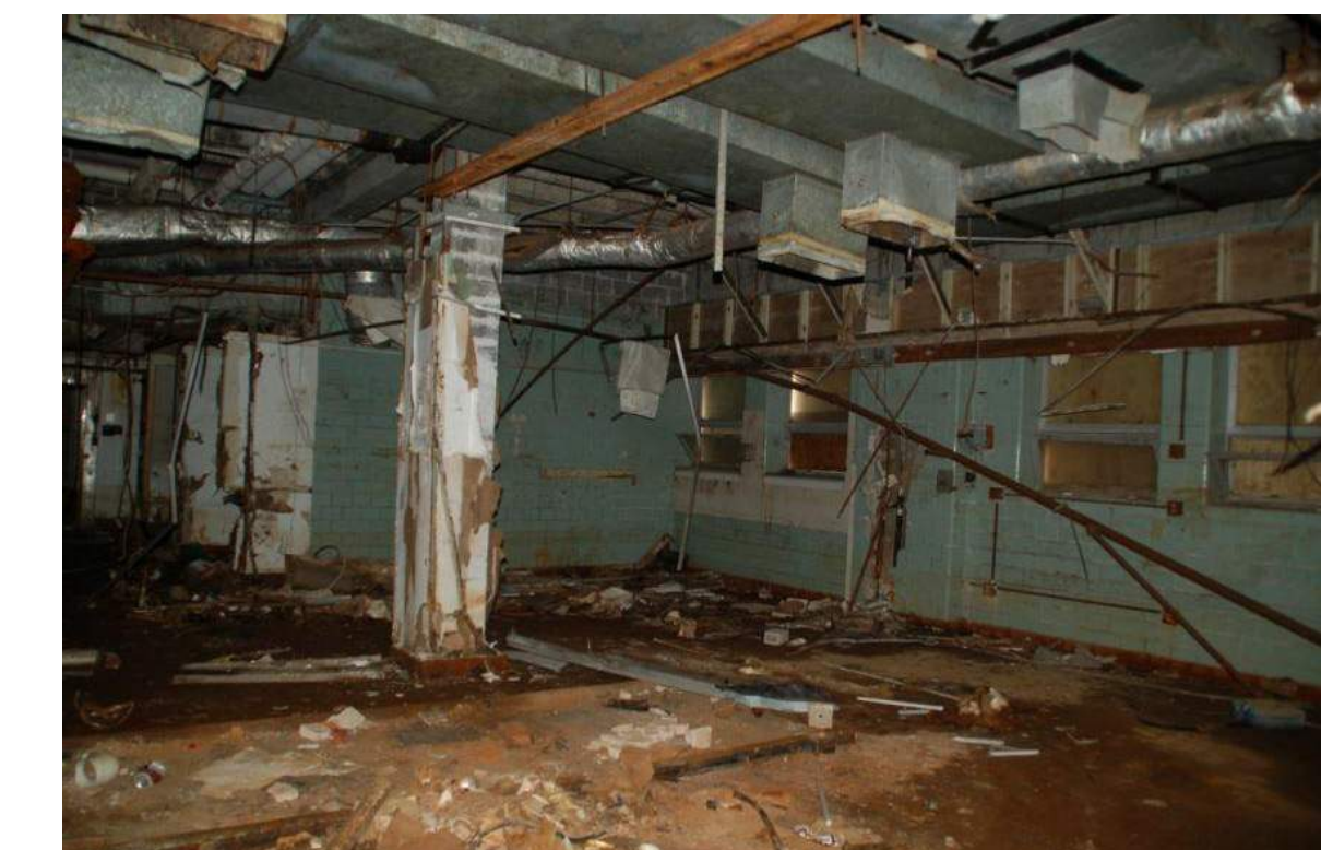
2 INTERIOR - BASEMENT - ORIGINAL HOSPITAL: KITCHEN GLAZED MASONRY WALLS TO REMAIN ON INTERIOR AND EXTERIOR WALLS. SALVAGE ANY LOOSE BLOCKS FOR RE-USE.
