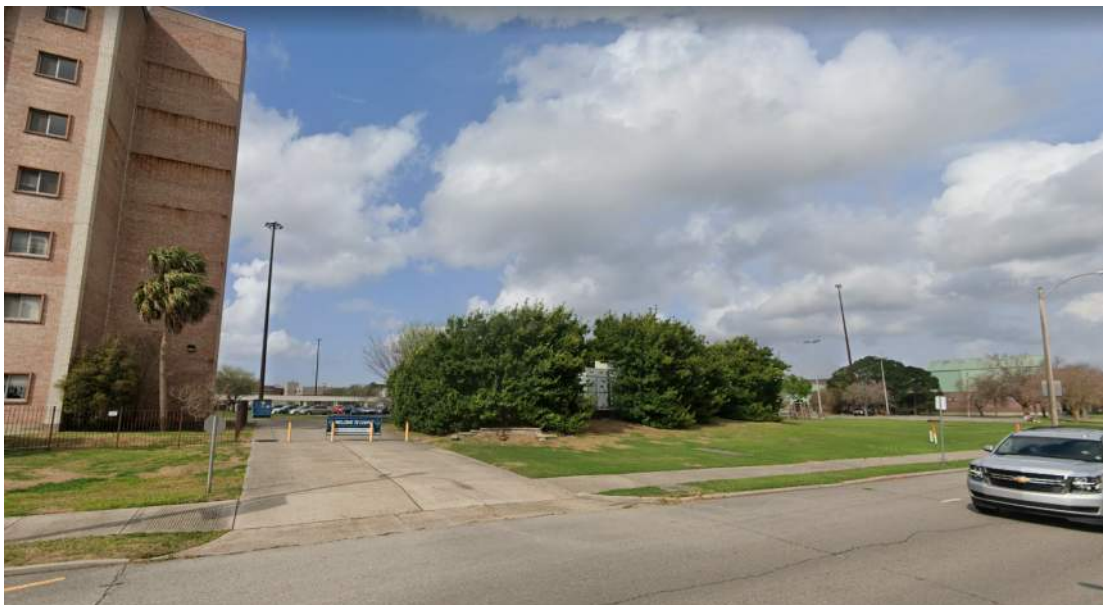
View of existing electrical substation (behind plantings) from Leon C. Simon Dr. (Bienville Hall on left side of photo to be demolished by UNO prior to Hynes construction.)
