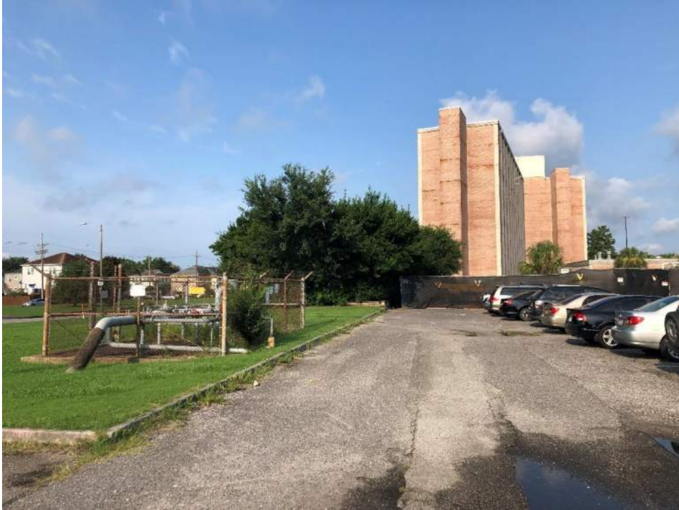
View of existing electrical substation (behind plantings) and gas manifold to remain.
