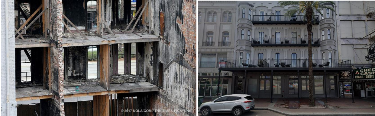
Figure 6. Damage from a fire at 1016 Canal Street in 2016 (left) and the rebuilt residential building currently operated at the address (right). Photo courtesy of Times-Picayune/NOLA.com.
