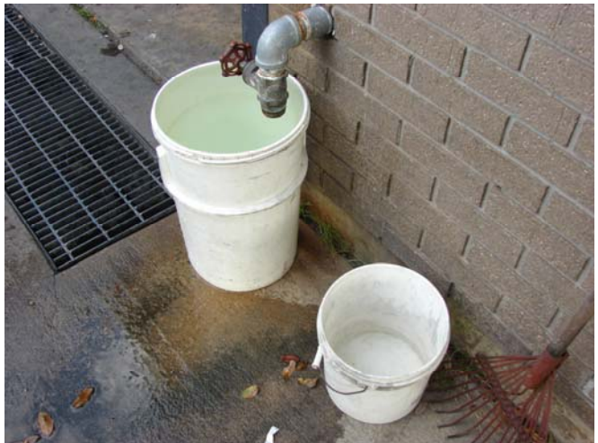
Figure 7. Leaks and standing water were a reoccurring problem that contributed to rodent infestations.
