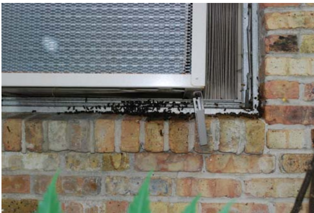
Figure 31. Honey bee colony in window air conditioning unit at residence in Algiers.
