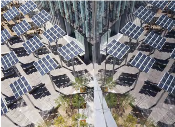
Solar Panels, City of Las Vegas City Hall
