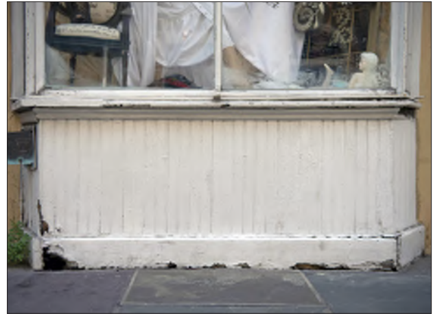
Wood in contact with the ground is more susceptible to damage from storm water, termites and fungi, requiring more frequent maintenance. The larger opening can also allow rodents and pests to nest under the display window.
