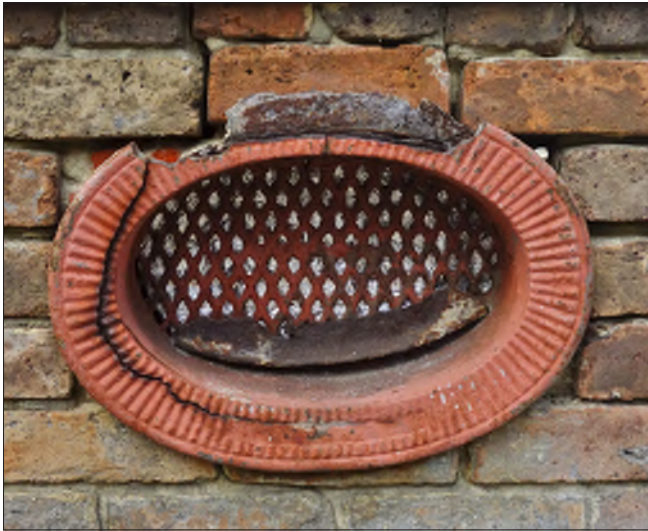
The foundation vent is cracked and rusting. The grille has been blocked from behind reducing air circulation in the crawlspace. Also note the loss of mortar at the brick joints.
