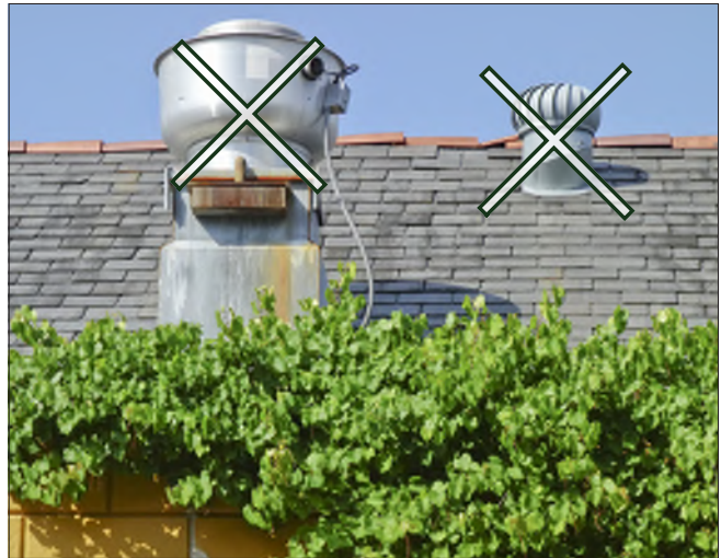
The restaurant vent (left) is located within the building envelope; however, it is visually prominent and, therefore, not appropriate. The turbine ventilator (right) is also not appropriate in the Vieux Carré.
