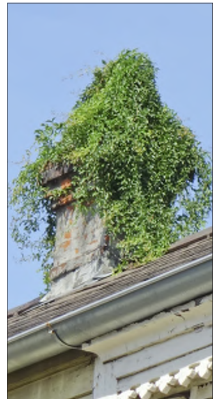
The vines on the chimney may clog the flue and dislodge the mortar.
