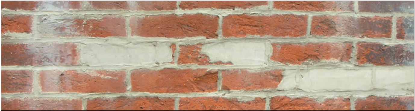
The rough texture and uneven surface suggest that an aggressive cleaning method was used. Stucco patches have replaced bricks and efflorescence, a white powdery substance, can be seen on the surface.
