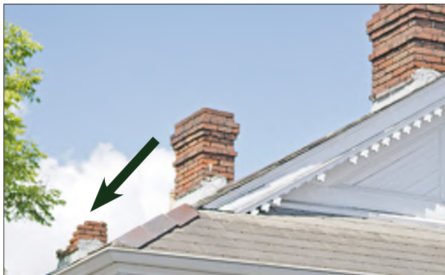
The rear chimney has collapsed and there is significant mortar loss at the remaining two chimneys.
