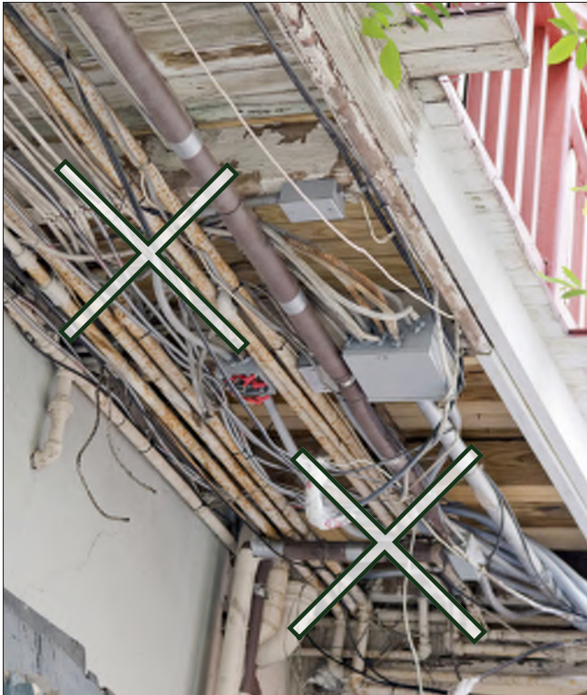
Exterior lighting and/or a security device typically requires the installation of wiring. As more wiring, piping and conduit is added, a potentially hazardous condition is created and the overall appearance may become cluttered. Abandoned wiring, piping and conduit should be removed.
