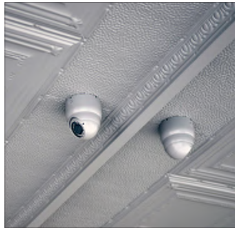
These dome-style cameras are mounted under a projecting canopy. Their housings are painted to match the canopy, minimizing their visibility.
