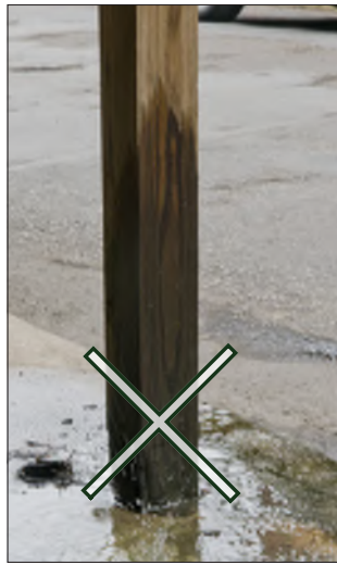
The base of this wood post is in constant contact with moisture and is rotting.
