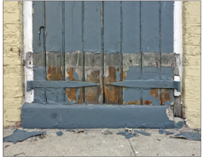
Improperly maintained paint along the bottom of the shutters leaves them susceptible to damage from moisture, termites and other pests.
