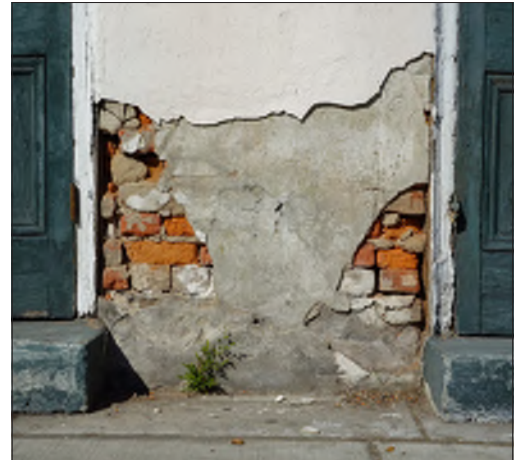
The cracked and missing stucco reveals loss of mortar as well as brick damaged from water infiltration.
