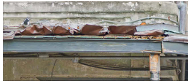
The edge of the roofing at this gallery is bent and not secure. A strong storm winds could peel the roof off of the building.
