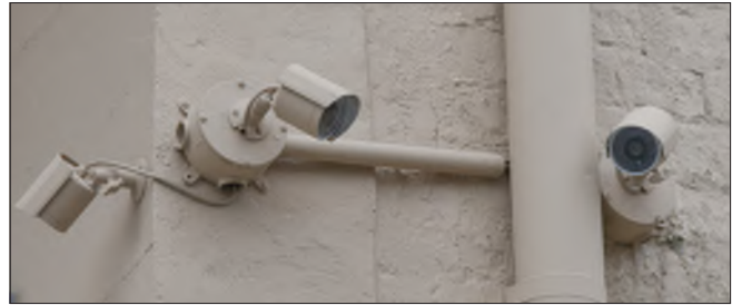
The vertical portion of the wiring is concealed by the downspout. The remaining conduit, junction boxes and cameras are painted to match the wall surface.
