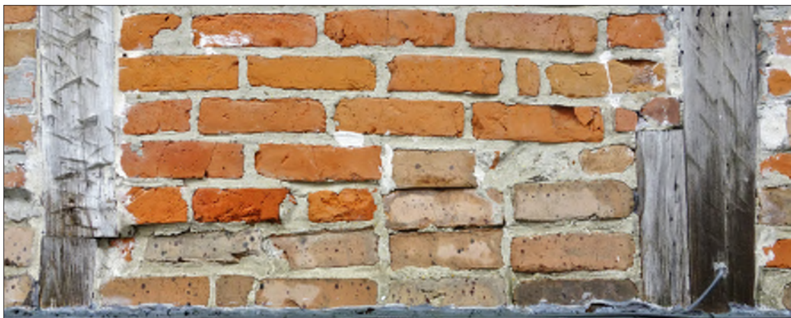
This brick-between-posts exterior wall, now exposed to the elements, was designed to be protected with a coating of stucco. Without this layer, the soft brick substrate quickly deteriorates. Wood repairs and replacement bricks are evident.
