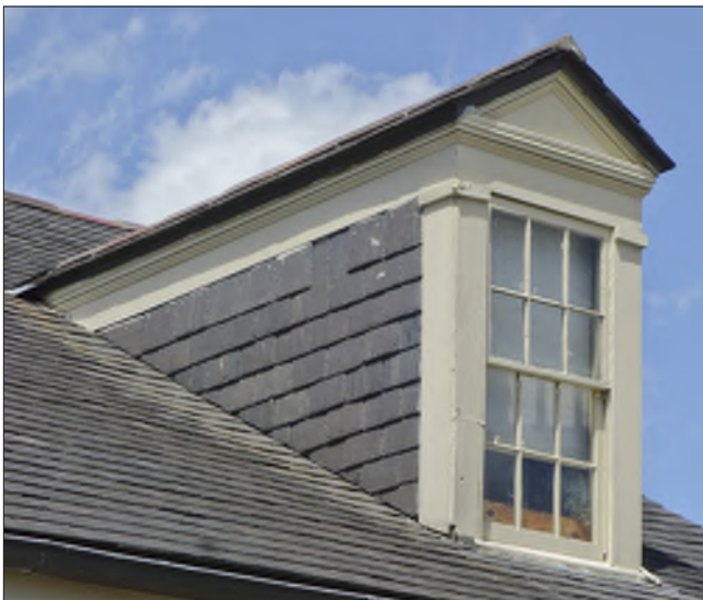
This dormer has a defined pediment, a triangular gable end, reminiscent of classical detailing. One slate is missing at the cheek wall, or side wall, and should be replaced.
