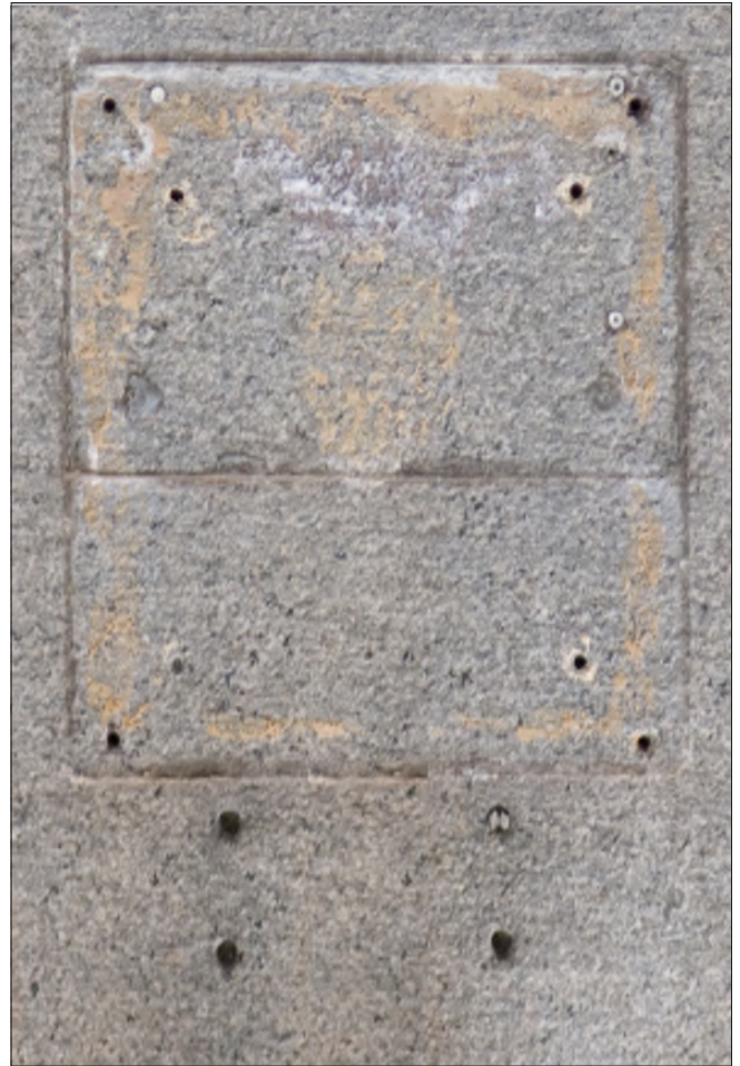
Numerous holes have been drilled into the face of this granite pier and several abandoned fasteners still remain. Fasteners should be removed, existing holes reused for future signs, abandoned holes filled and the stone surface cleaned. (Refer to Guidelines for Masonry & Stucco.)
