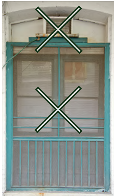
Exterior screens obscure the view of historic window and door features. The air conditioner unit and an infill panel have replaced the former transom window. Obscuring or removing a historic element or feature is not appropriate in the Vieux Carré.
